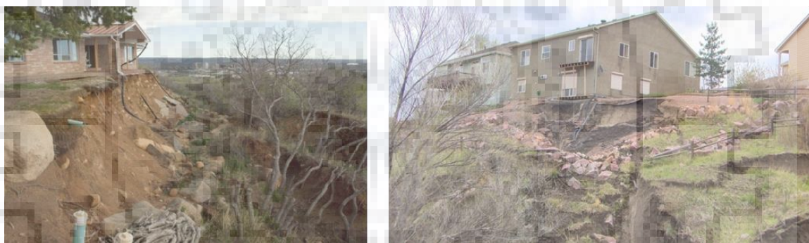
Figure 1.1 Building location and foundation failure on slope
