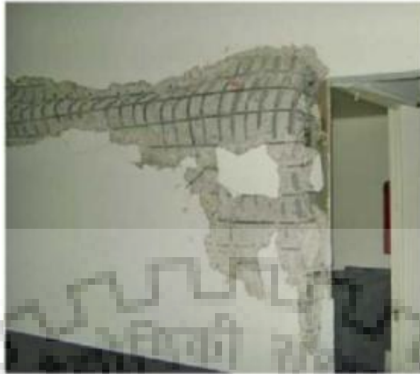
Figure 2.2 Damage at wall discontinuity [17]
