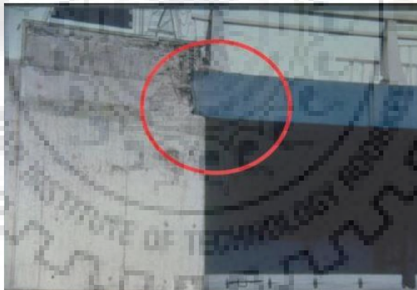
Figure 1.4 Pounding damage at the abutment 1995 Kobe earthquake (Brando 2012).
