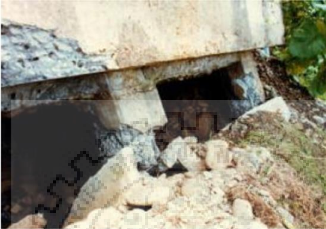
Fig. 1.4 Damage to front batter pile of Rio Banano bridge (Priestley et al. 1991)
