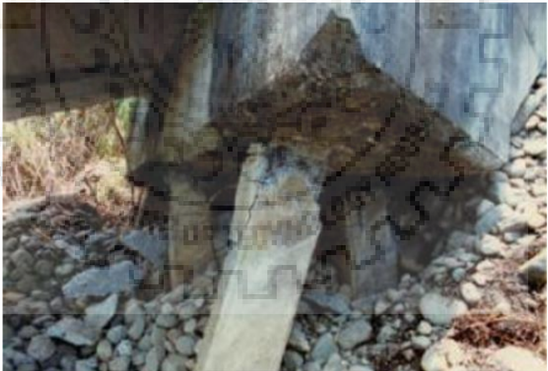
Fig. 1.3 Failure of Rio Vizcaya bridge (Priestley et al. 1991)
