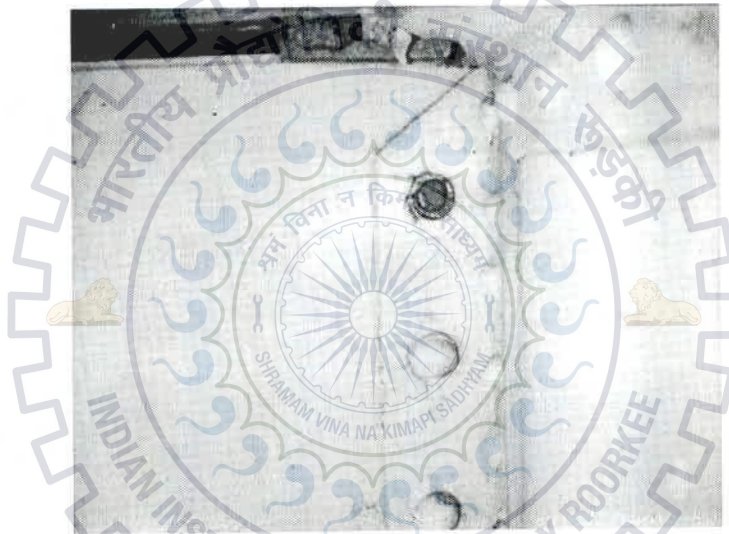
Figure 3.6 – Failure of rivet shank under fatigue (Åkesson, B., 1994)
