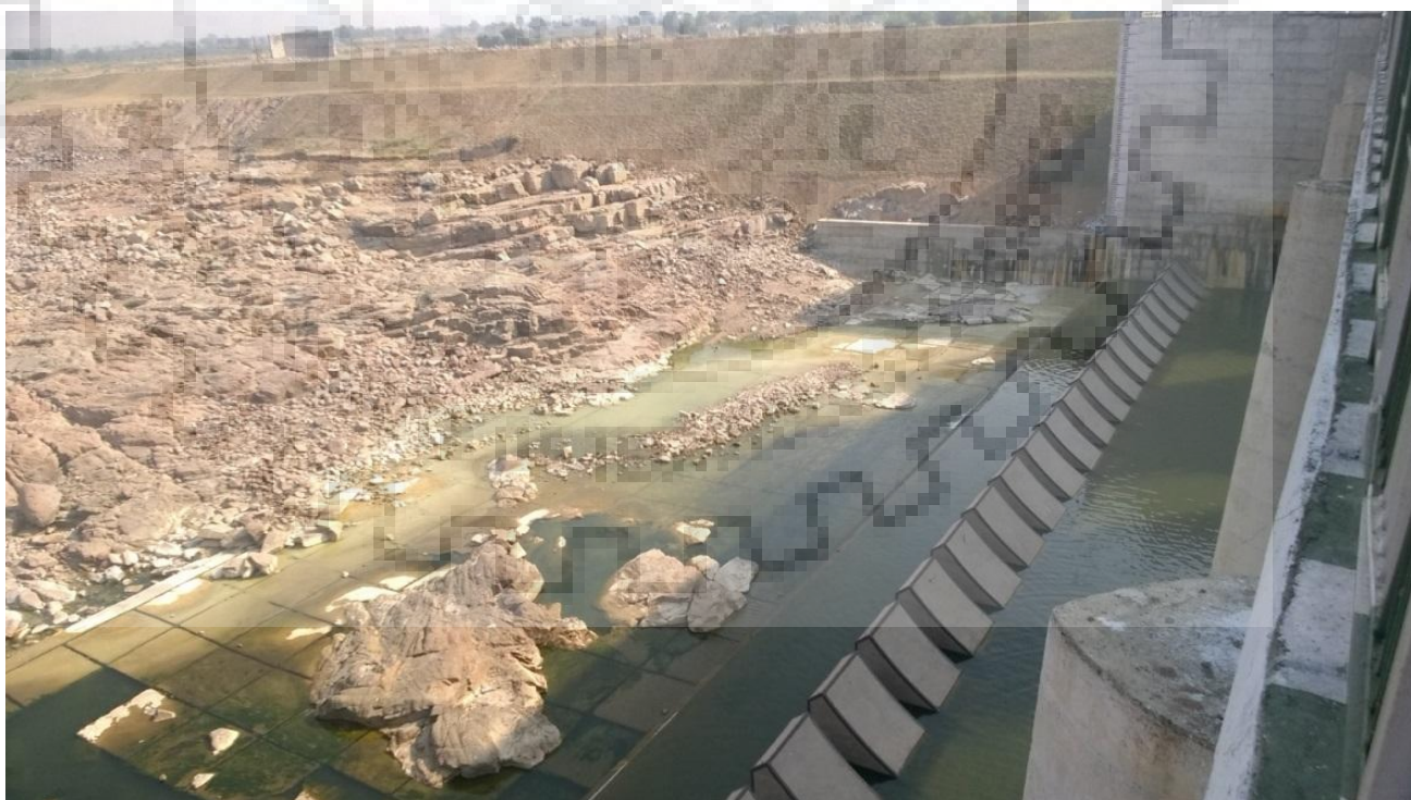
Place: Energy dissipators in Lahchura Dam near Mau-Ranipur Latitude: 25°13'41.8597"N Longitude: 79°13'50"E Elevation: 169 m
