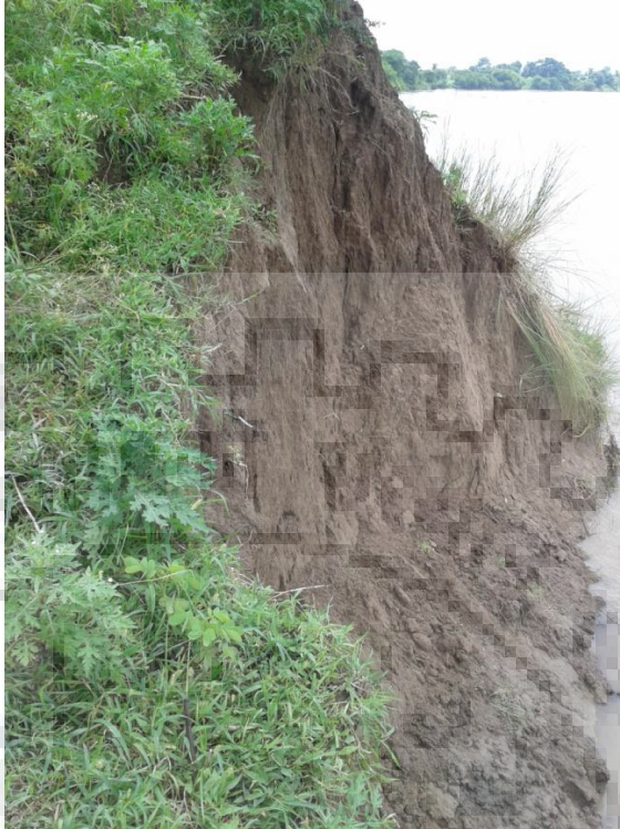
Place: Basoda-Ganj Village- cutting of river bank by Betwa River water flow near Rapta pul Latitude: 23° 52' 41.0", Longitude: 77° 55' 05.6", Elevation: 400 m
