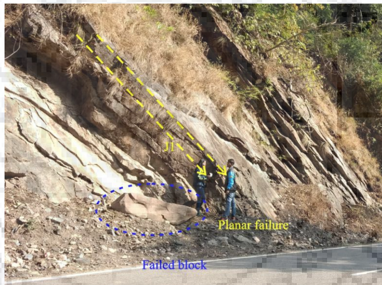
Figure 3.10: Daylighting conditions offering a planar mode of failure due to joint set J1 at slope S8 and failed blocks at the toe portion of the slope
