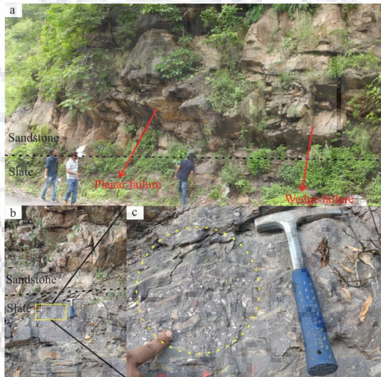
Figure 3.6: Field photograph depicting the condition of rock mass at slope S4 (a) Showing the joints forming a wedge and planar sliding (b) Lithological contact between Slate and Sandstone (c) Inset image showing clast at lithological contact
