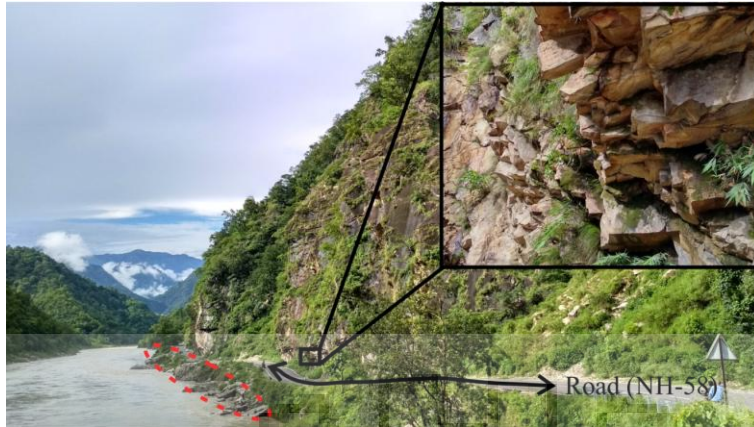
Figure 3.23: A panoramic view at slope S10 along NH-58 during monsoon season showing the level of water in the Ganga River, causing toe cutting and seepage through joints and Inset view is depicting jointed & blocky rock mass conditions at slope S10
