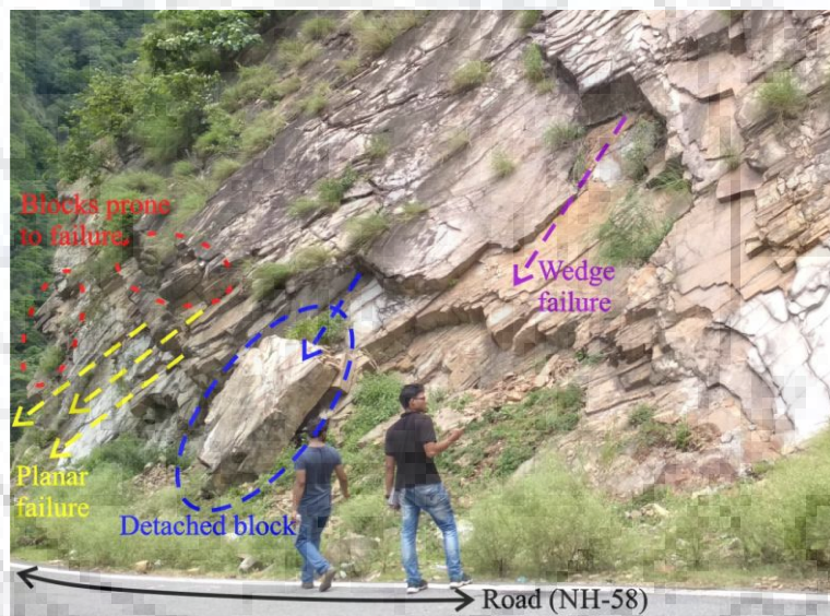
Figure 3.18: Failed blocks and potential rockslide for different modes of structurally controlled failures at slope S16
