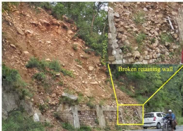
Figure 3.29: Debris material with mixed clast size at location L5 and inset image showing damaged retaining wall
