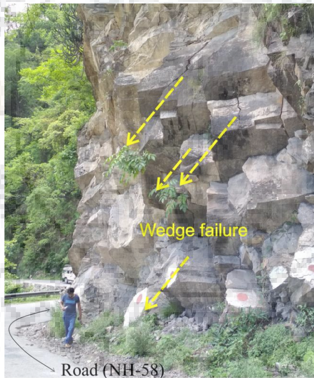
Figure 3.19: Blocky rock mass having significant potential for wedge failure at slope S17
