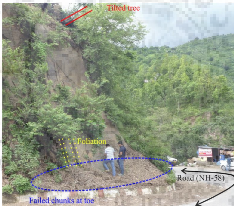
Figure 3.9: Weathered and soft rock causing failure of small chunks and tilted trees indicating deformation within rock mass at slope S7
