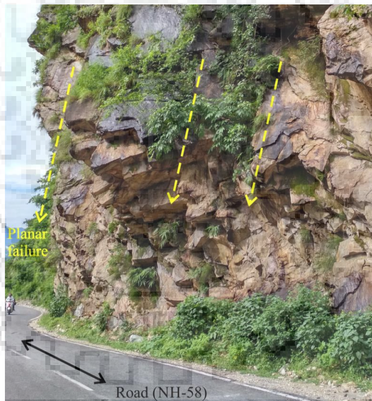
Figure 3.12: Rock mass having persistent joints offering planar failure followed by rockfall at slope S10
