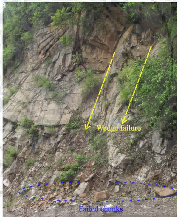
Figure 3.20: Failed chunks and condition favorable for wedge failure at slope S18
