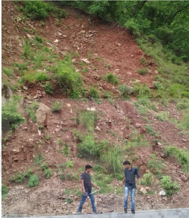
Figure 3.30: Failed debris at location L6 along NH-58
