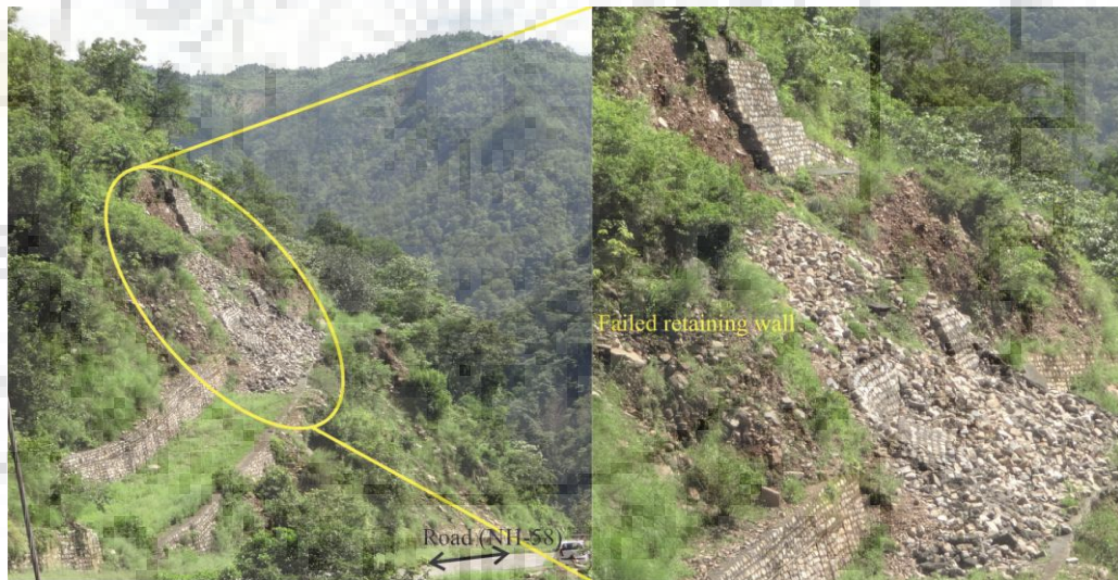
Figure 3.31: Debris slope at location L7 along NH-58 and inset image showing the failed retaining wall
