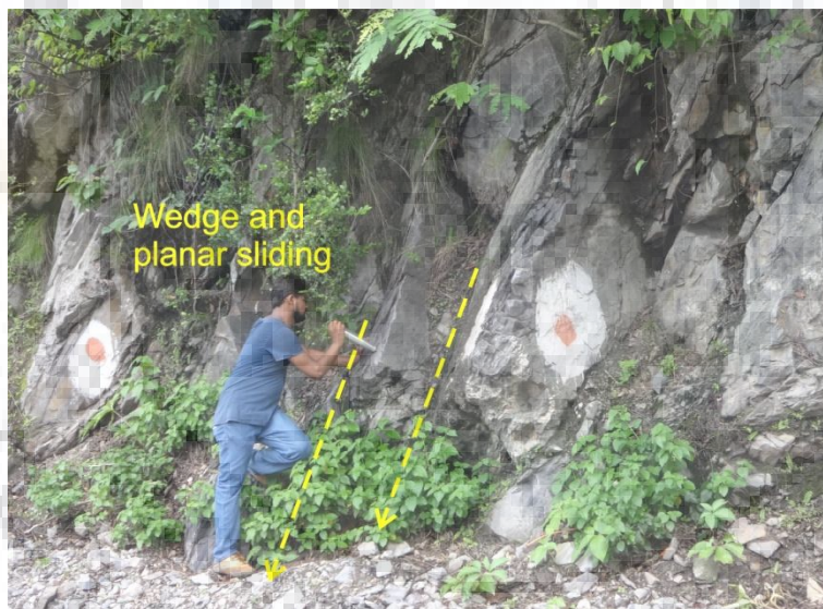
Figure 3.21: Adversely oriented discontinuities causing wedge and planar sliding at slope S19
