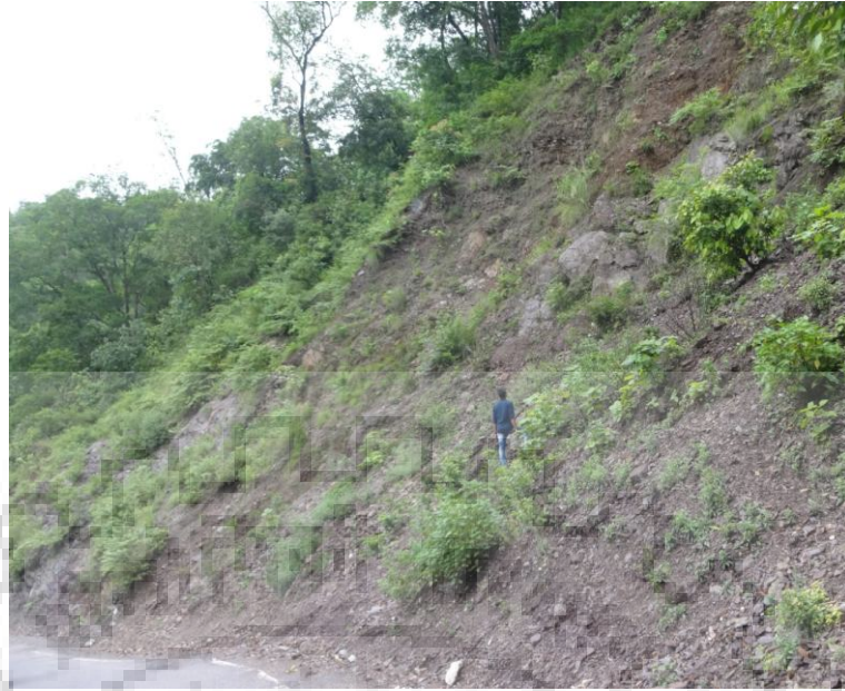
Figure 3.26: Panoramic view of road cut debris slope at location L2 along NH-58
