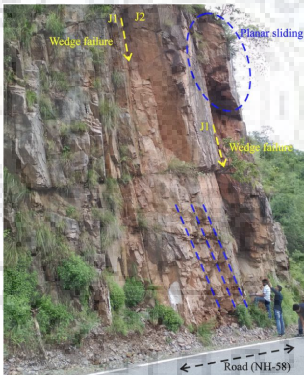
Figure 3.13: Adversely oriented joints favoring planar and wedge sliding at slope S11
