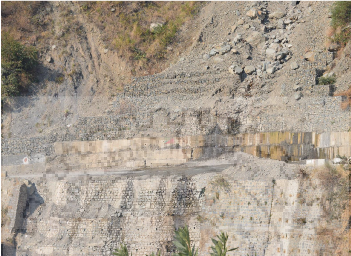
Figure 1.2: Destroyed retaining structure at the toe of the Lakhwar Dam Top Landslide (Photo taken on 14 th January,2018)
