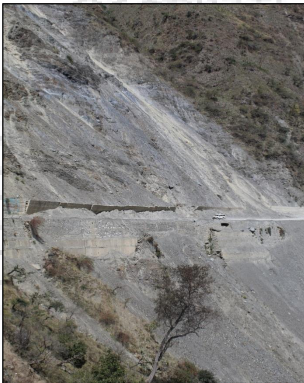
Fig. 5.10 (a): Landslide Observed at 30°33.817' N, 77°51.081' E
