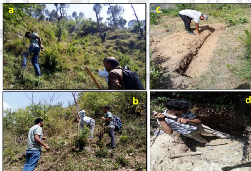
Figure 8.2: Intervention work in the springshed a) Recharge area identification, b) Mapping for slope, c) Contour Trench and d) Percolation Pit
