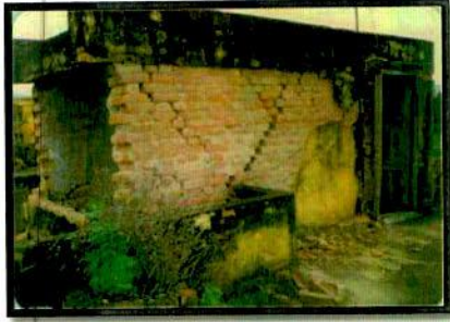
Figure 23: Damaged building at Munger during 1988 Bihar-Nepal Earthquake
