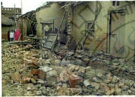
Figure 6: Damaged masonry house in Madhubani, Bihar
