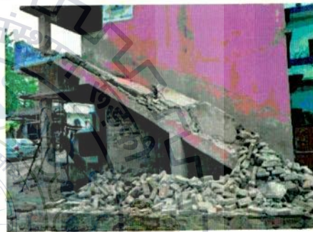
Figure 7: Damaged school building in Motihari, Bihar
