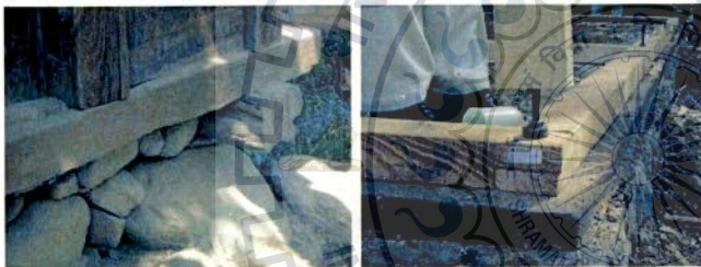
Fig.3.28. Evolution in connection of plinth to the foundation (Source: World Housing Report #146)
