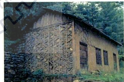
Fig.3.25. Dhajji dewari house showing bracing, masonry and mud plaster (Source: World Housing Report #146)
