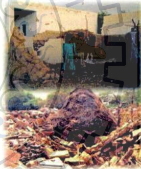
(Choudhary et. Al 2002) Fig.3.8. Collapse of adobe wall Bhunga houses
