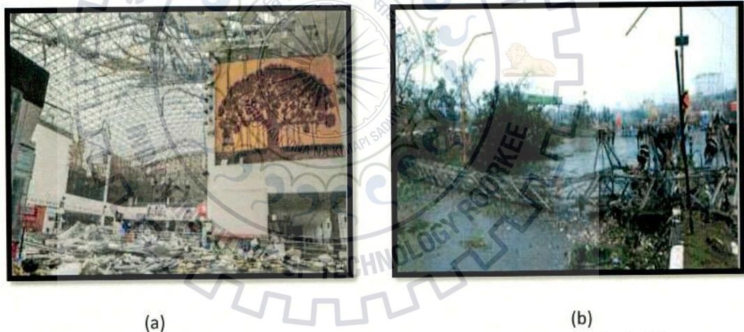
Figure 3.2: Damage due to winds during VSCS Hudhud (a) Damaged roof of Vishakhapatnam Airport (b) The collapsed telephone tower near Visakhapatnam (Source: IMD, 2014)
