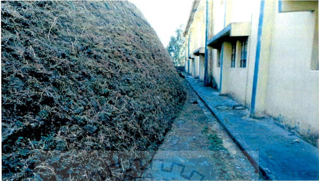
Fig 3.3: Back view of Block II showing soil retained by high retaining wall
