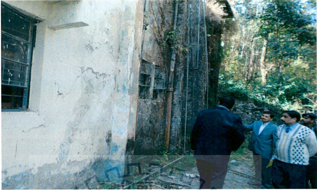
Fig 3.8: Damages due to dampness and appearance of cracks in column
