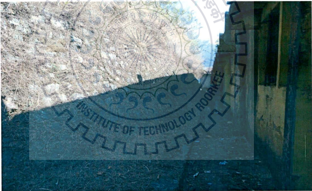
Fig 3.9: Damages in column due to movement of retaining wall
