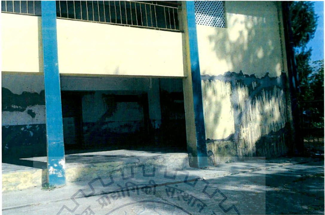
Fig 3.4: Damage in masonry infill panel of classrooms and exterior wall
