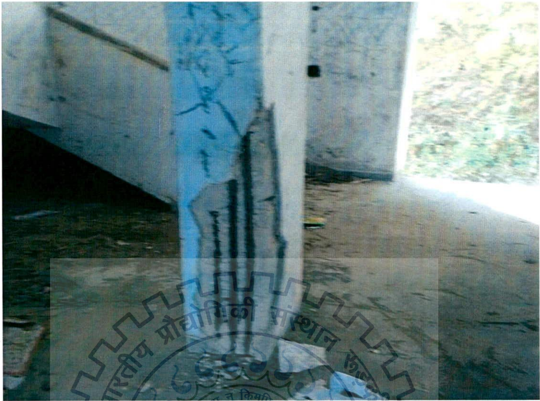
Fig 3.6: Spalling of concrete cover showing missing stirrups
