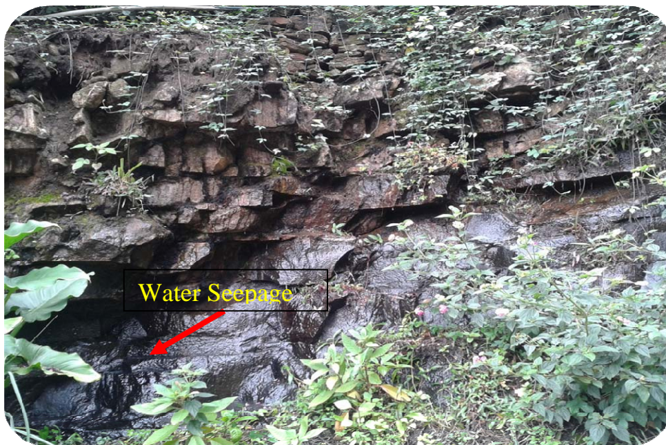
Fig 2.14 Highly dissected rock exposure seen along the Observatory Road showing water seepage along the joints
