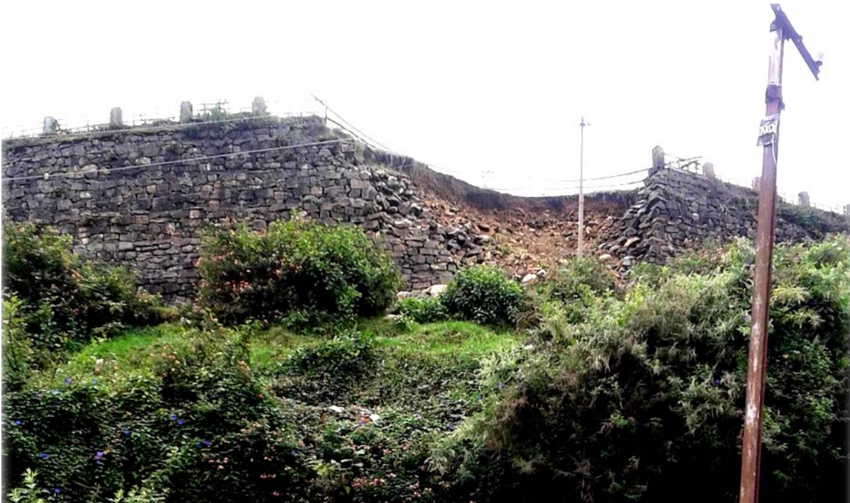
Fig 5.31 Collapse of retaining wall at Observatory road
