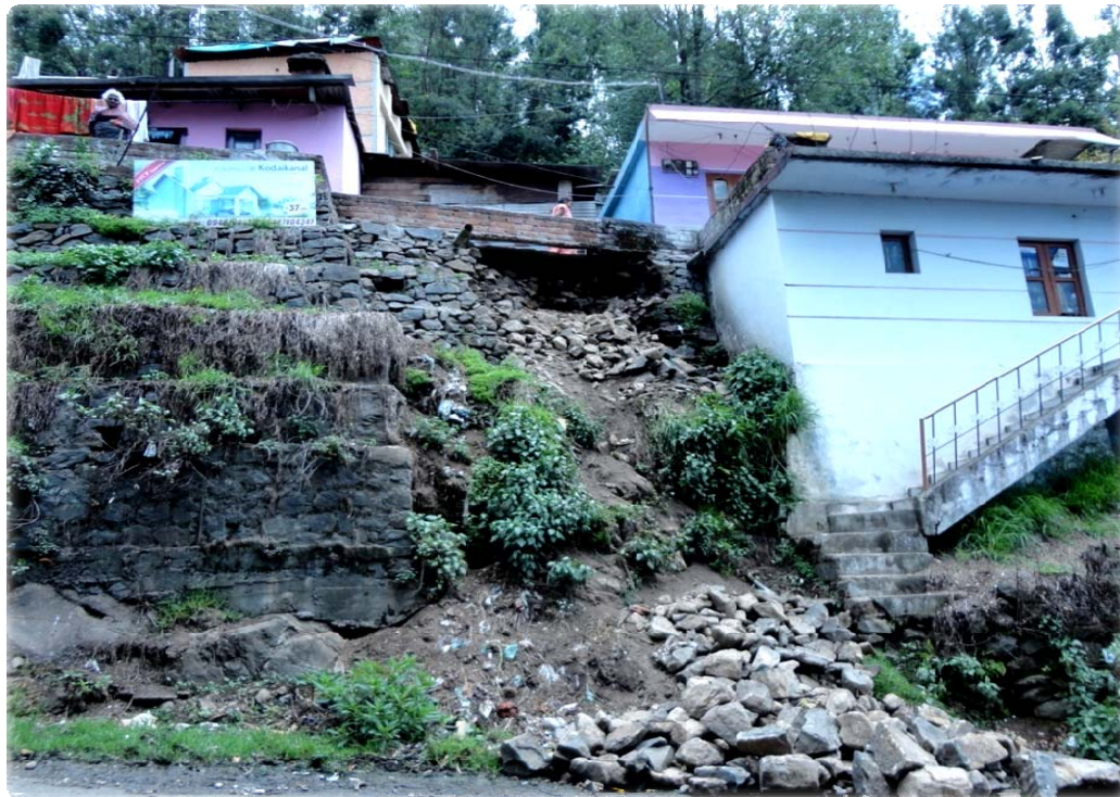
Fig 5.30 A small slide on the urbanized slope of the Pudukkad slope
