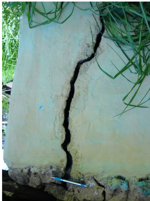
Fig. 2.9 Crack found in a house at Gandhipuram Slope
