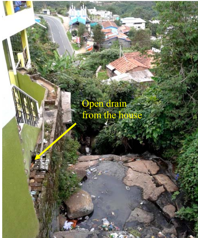
Fig 5.14 Improper waste water management seen at the slope
