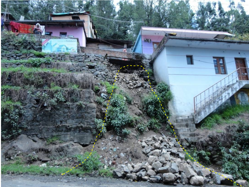
Fig 2.15 A slide along the Observatory road, below the houses
