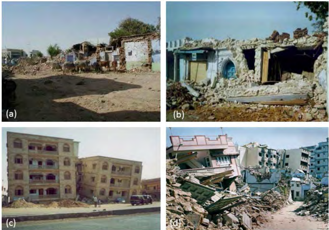
Figure 1.6: (a) Most stone houses in the old town of Bhuj collapsed, (b) Damage to cut stone and lime mortar masonry building in old Bhuj, (c) Taksila Apartments, Bhuj. Both 5-story buildings collapsed due to soft story effects, (d) Damage to the RCC building ( http://peer.berkeley.edu/pdf/2713_Other200104GujaratEQTR0101.pdf accessed on 28-04-2017).
