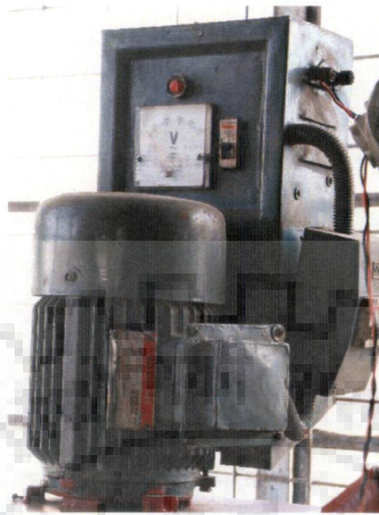
Fig.4.4 Photograph of generator set
