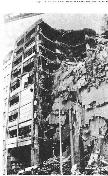
Fig. 1.13: Katrantzos department building in Athens after the 1980 fire (Beitel and Iwankiw 2002)
