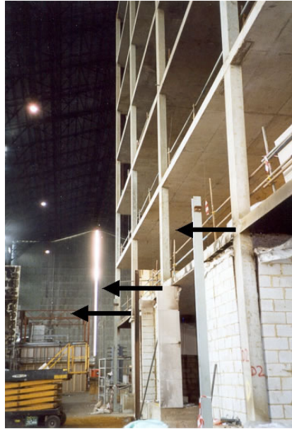
Fig. 1.11 - Picture showing lateral displacement of external columns (Bailey 2002)
