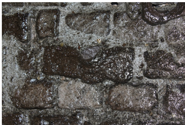
Fig. 3.14: Solidified molten mass from masonry walls
