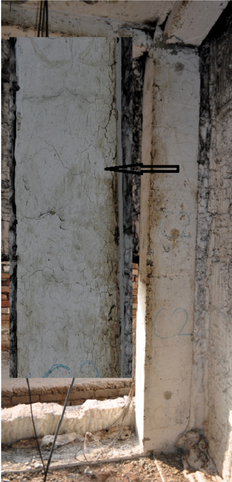
Fig. 2.41: Fire damage in Column C2
