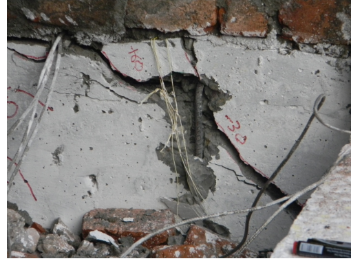
Fig 3.6: Shear failure in beam B3.
