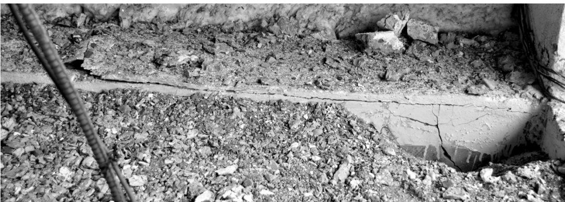
Fig.2.45: The delamination of the cover concrete in Beam B3
