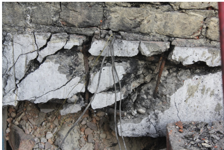
Fig 3.28: A closer view of the beam B1 showing damaged portion
