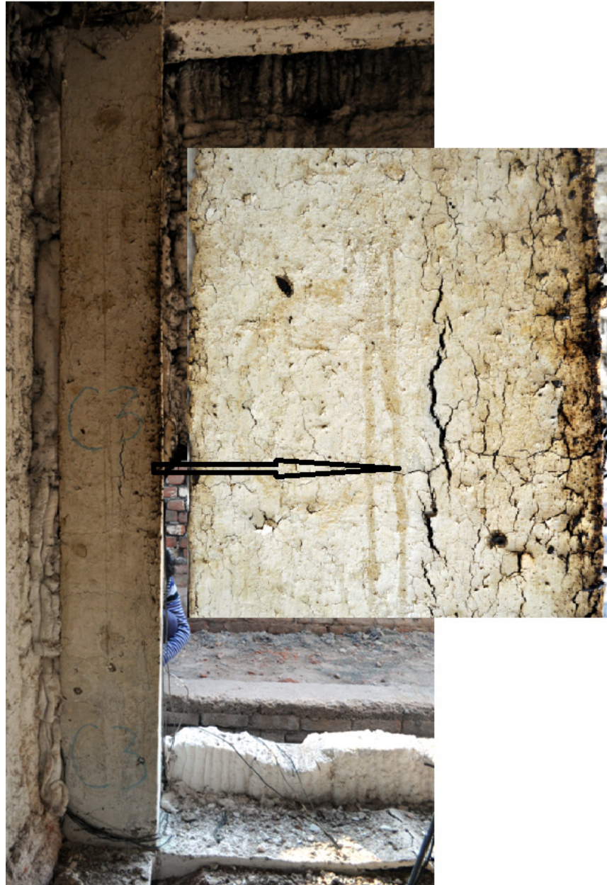
Fig.2.42: Fire damage in Column C3
