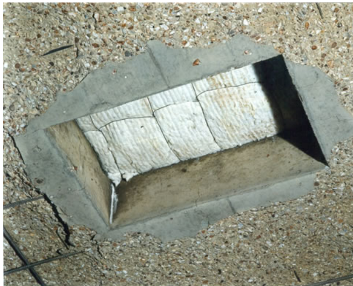
Fig. 1.10 - Picture showing spalling around service hole (Bailey 2002)
