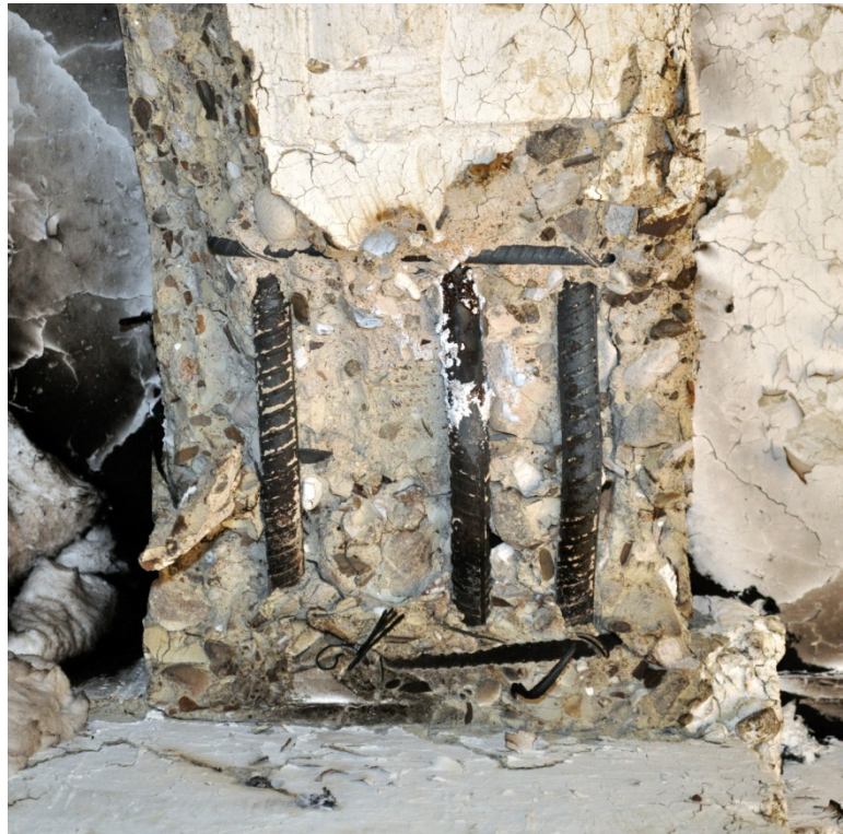
Fig. 2.47: Buckled reinforcement bars (Beam B7) exposed to direct flame
