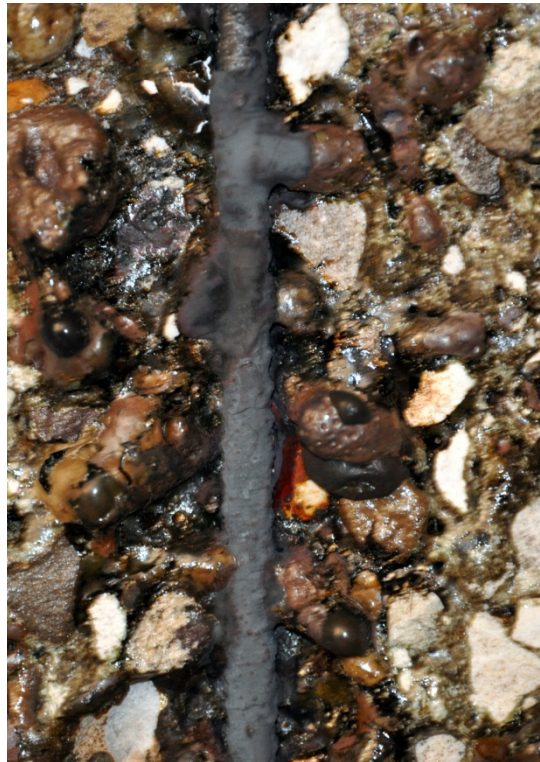
Fig. 2.50: Reduced cross section of the reinforcement of slab due to fire exposure.
