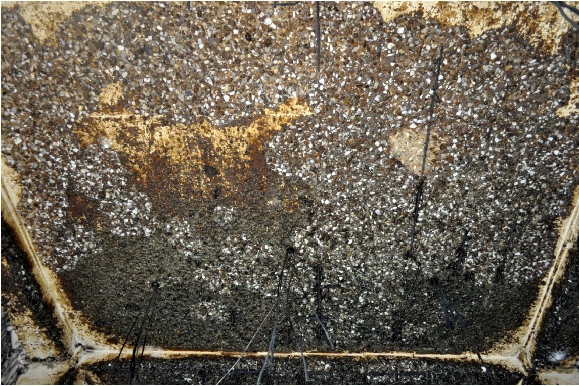
Fig.2.49: Spalling in slab
