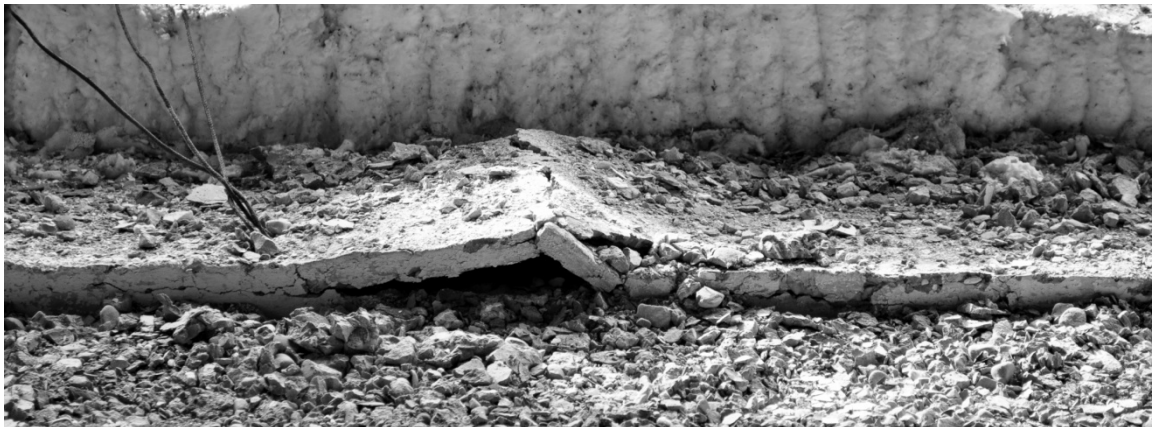
Fig.2.43: Delamination of concrete cover in beam B2
