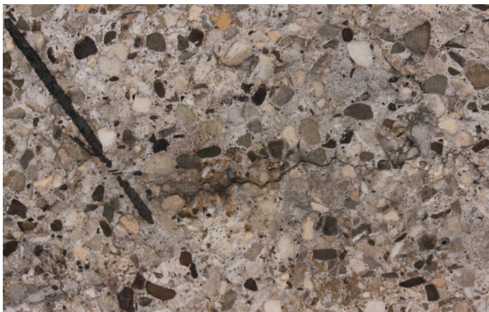
Fig.3.13: Exposed reinforcement in slab and the flexural cracks.
