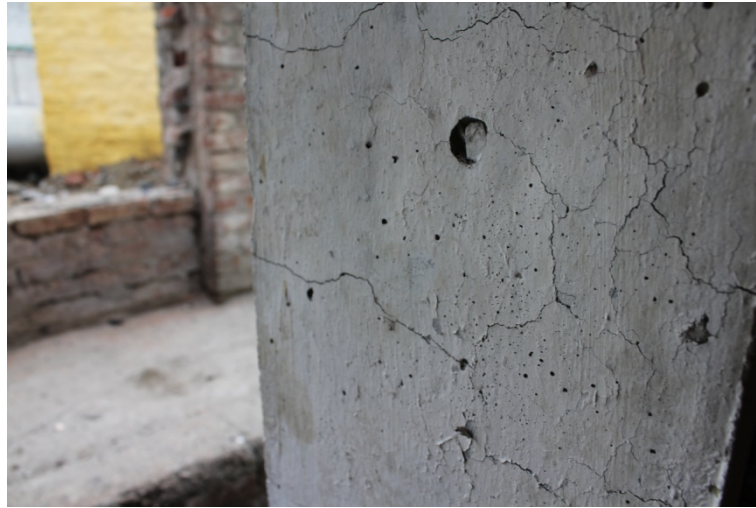
Fig.3.15: Thermal cracking in Column C2
