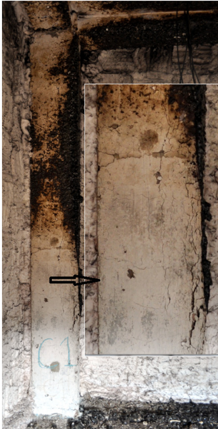
Fig. 2.40: Fire damage in Column C1
