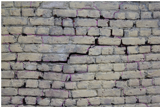
Fig. 3.4: A close up image of In-plane wall after the test
