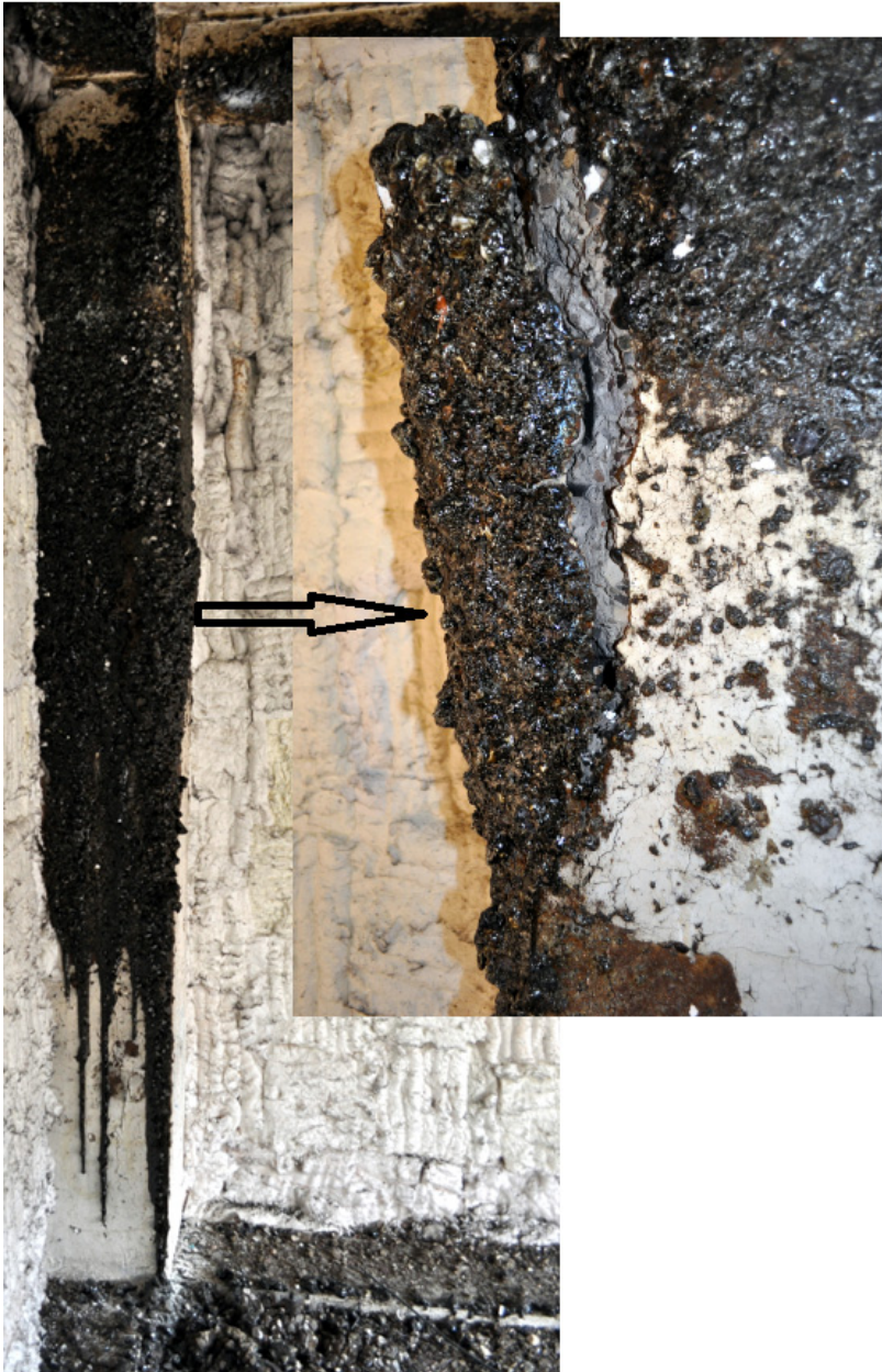
Fig.2.44: Fire damage in Column C4
