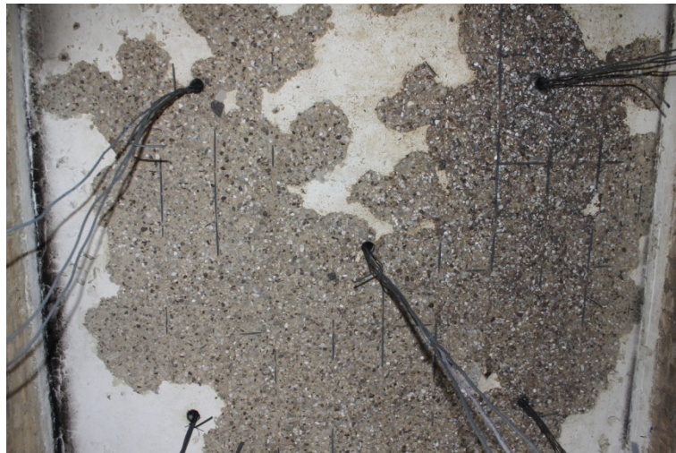
Fig. 3.11 Spalled soffit of the slab.
