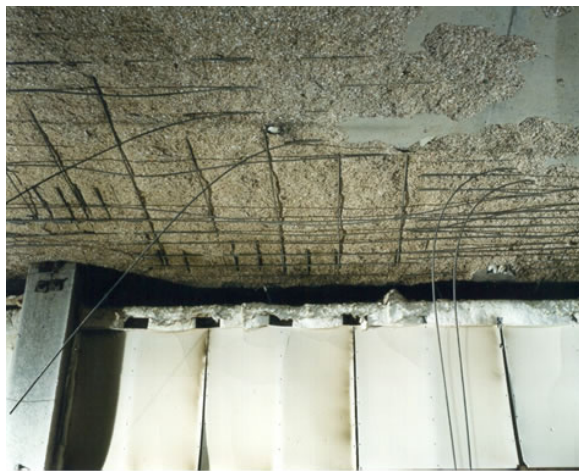
Fig. 1.9 - Picture showing extent of spalling of roof slab (Bailey 2002)
