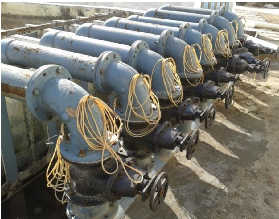
Figure 3.14 Close-up view of bend meters used to measure discharge of the model
