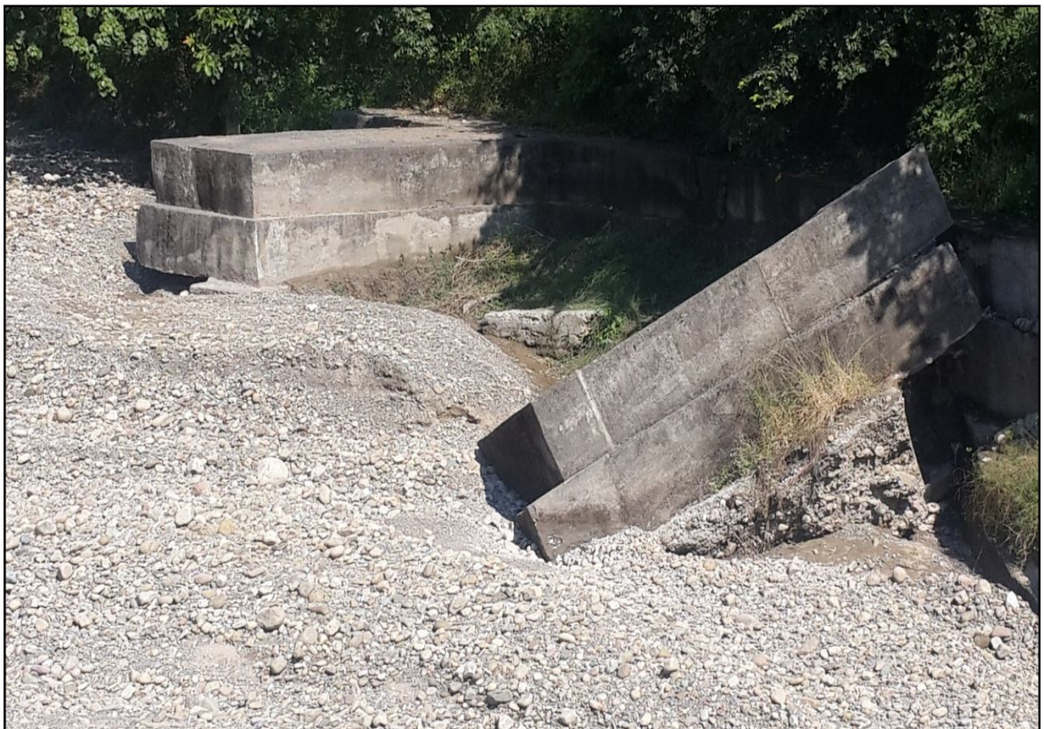
Fig. 1.4 Failure of Spur dikes at river Bhakhra near Haldwani, Uttarakhand (India)
