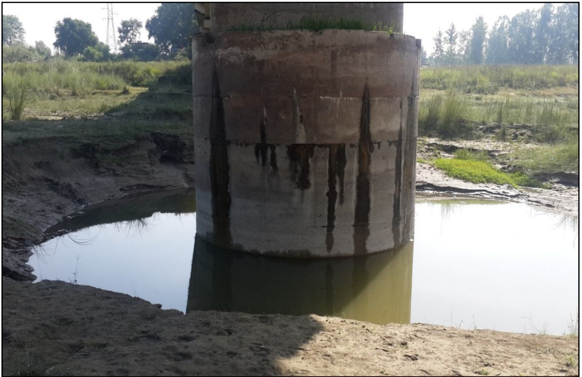
Fig. 1.2 Bridge pier scour at river Kosi at Kushinagar, Uttarakhand (India)
