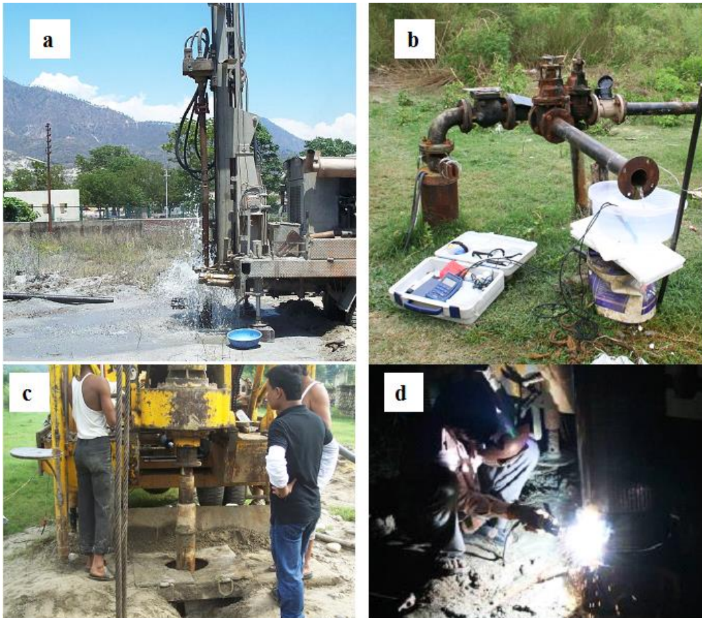
Figure 3.5 Srinagar RBF site. (a) Construction of production and monitoring well using ODEX method; (b) Pumping test; (c) Direct rotary technique; (d) Well assembly
