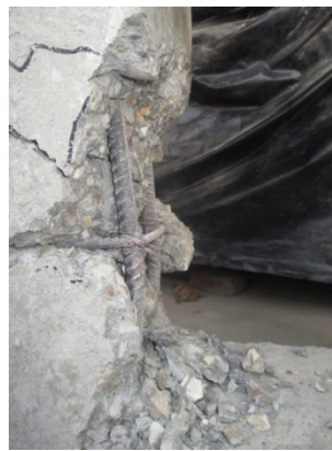
(b) Rebar buckling
