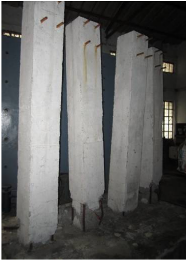
(a) Impaired column members
