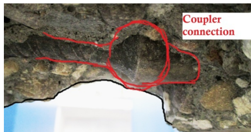
Figure 7.18: Coupler connection in CB 162 after specimen failure
