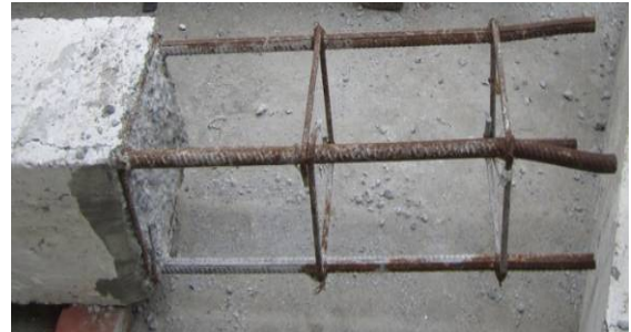
(b) Damaged concrete removed column
