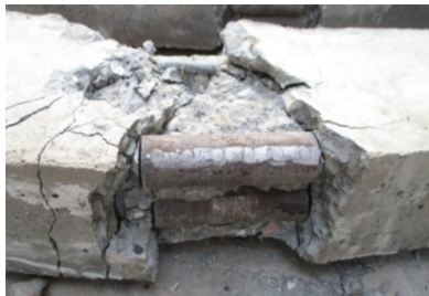
(a) coupler connection after failure
