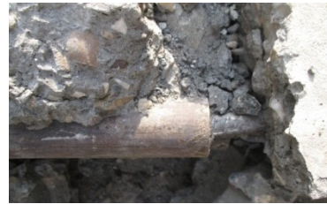
(b) Close-up view of connection
