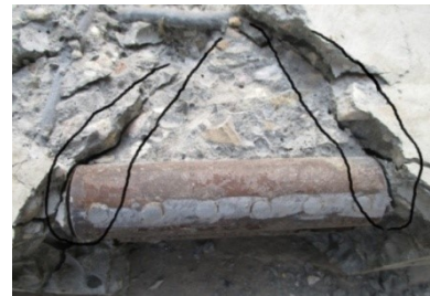
(b) Close-up view of connection
