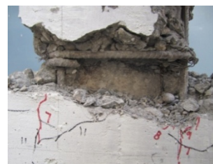
(b) Core cracking in SP 4
