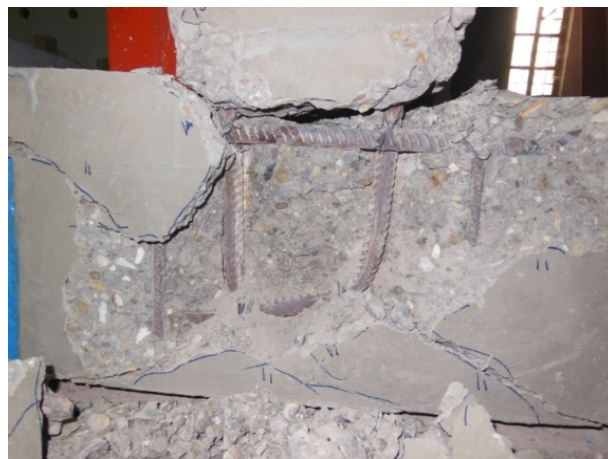
(b) Joint shear failure and beam-column connection failure
