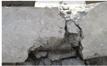
(a) coupler connection after failure
