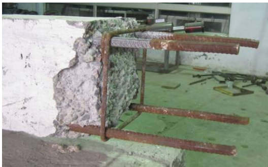
(c) Straightened buckled bar in column
