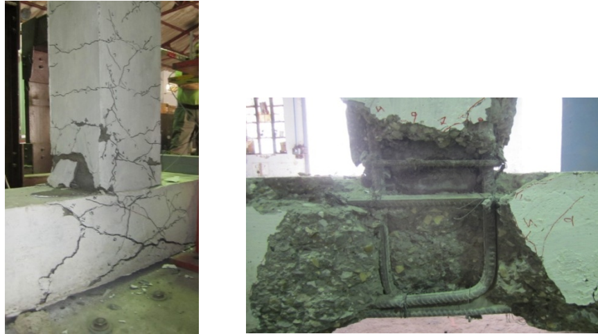
(a) Shear cracks widening (b) Joint concrete cover failure
