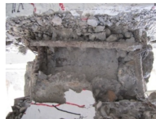
(c) Reinforcement buckling in connection SP4
