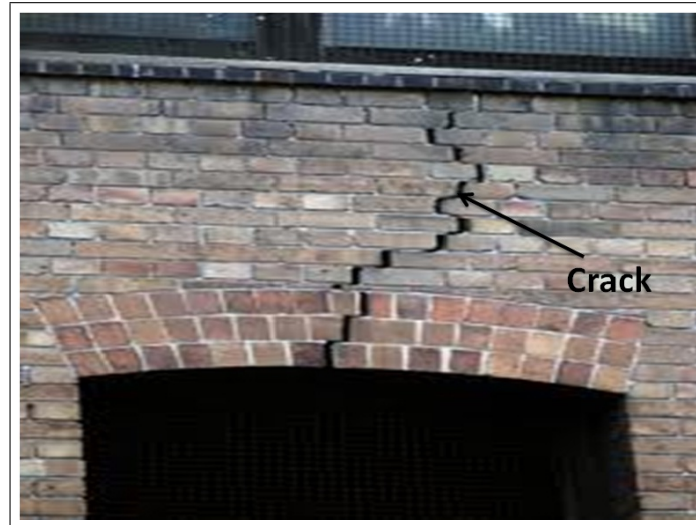
Figure 1.11: Crack in the wall
