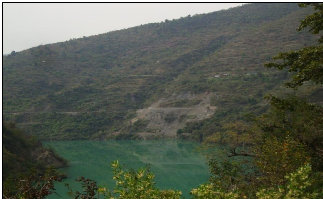
Plate 4.12 A View of Slope RBS12 Located 7.7 km d/s of Zero Bridge (near Phipalti village)
