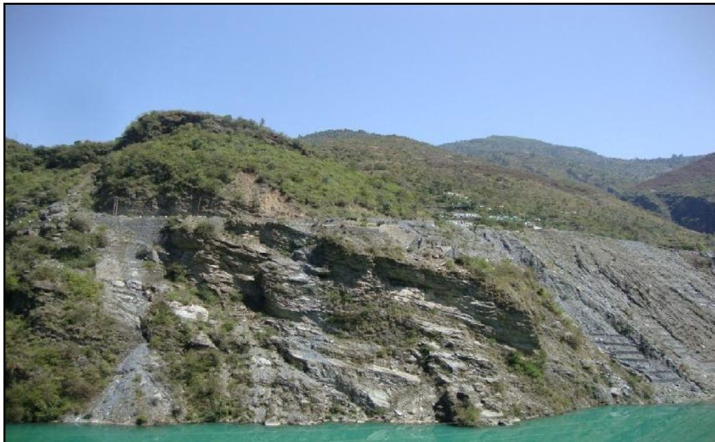
Plate 4.19 View of Slope LBS2 Located 900 m d/s of Zero Bridge (opposite of Marh Stream)
