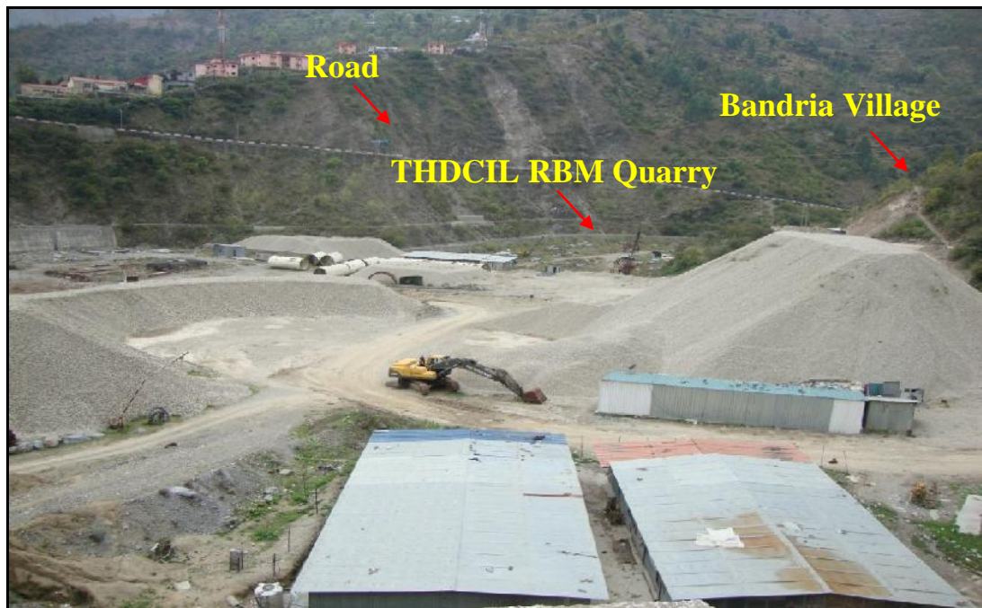
Plate 4.13 A View of Slope RBS13 Located 8.5 km d/s of Zero Bridge near THDCIL RBM Quarry near Bandria Village
