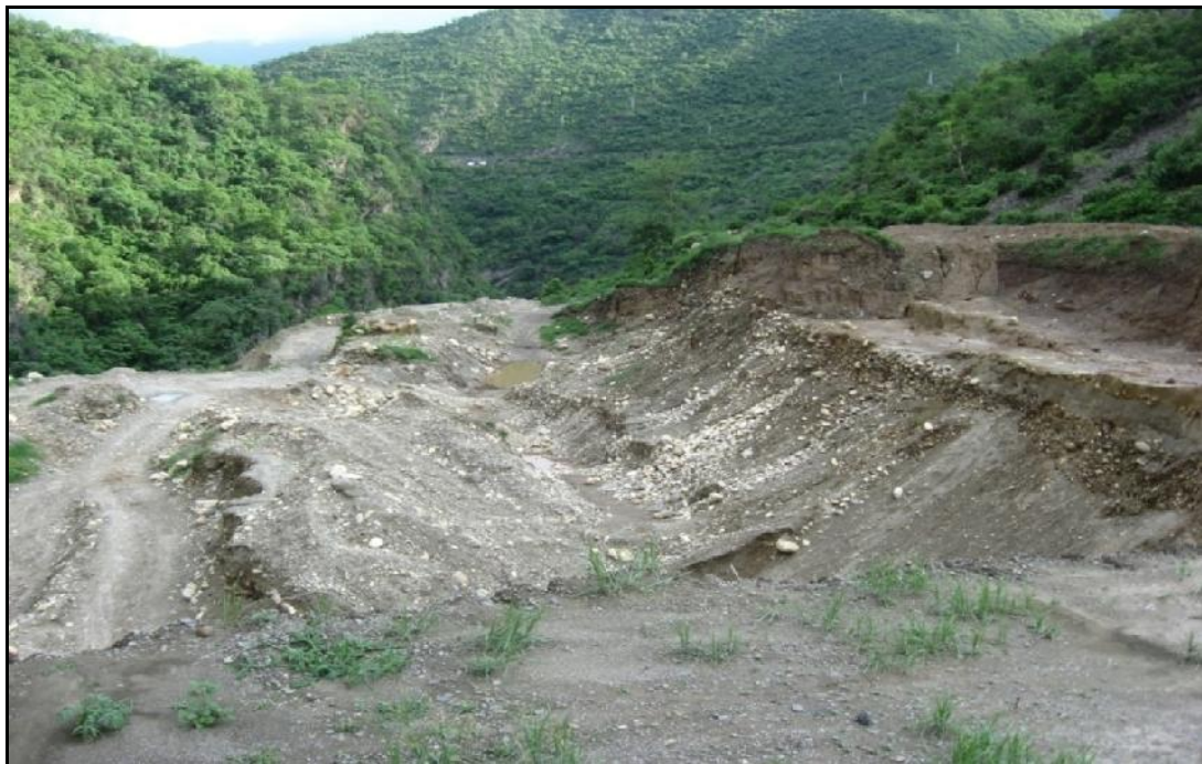
Plate: 4.9 A View of Slope Slope RBS9 Located 5.7 km d/s of Zero Bridge (near Quarry Site below Palam Village)
