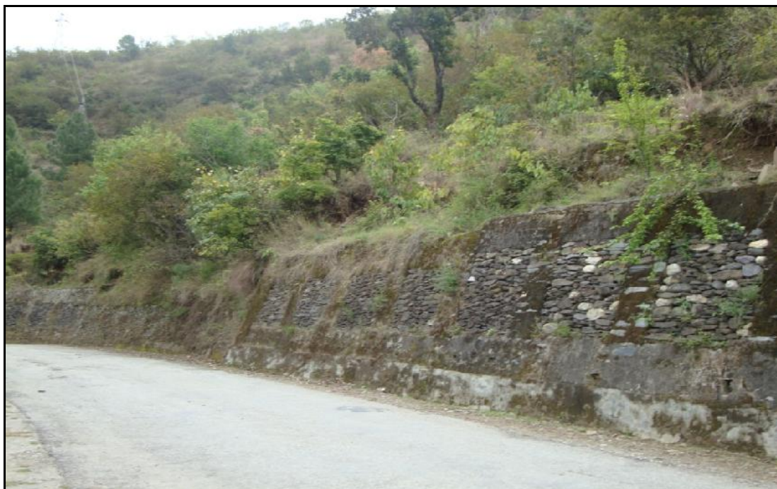
Plate 4.4 A view of Slope RBS4 Located 2 km from Zero Bridge (u/s of Dobra village)
