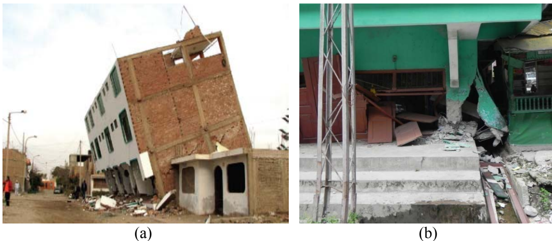
Fig. 3.6 Ground story failure due to torsional effect caused by irregular (asymmetric) ploacing of infills, during: (a) 2007 Peru earthquake (Johansson et al. 2007), and (b) 2011 Sikkim earthquake.
