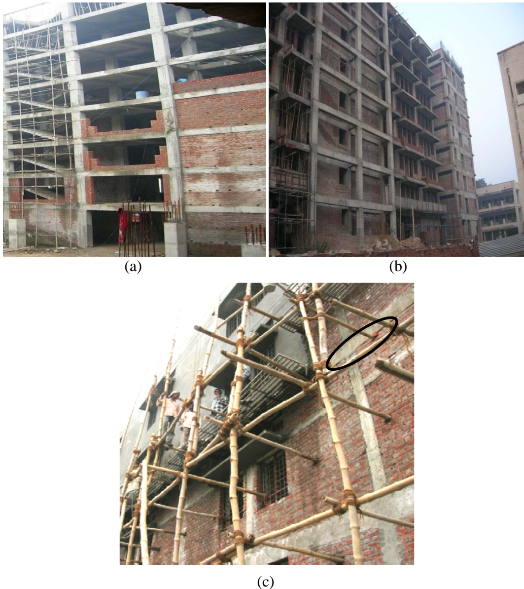
Fig. 1.1 Photographs showing typical construction sequence of an infilled frame building: (a) intermediate stage, (b) final stage of construction, (c) gap between infills and beam due to construction sequence of infilled frames.
