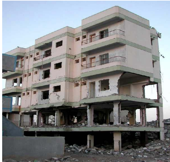
Fig. 3.5 Soft storey phenomenon due to out of plane failure of infills in bottom storeys, during 2001 Bhuj earthquake.
