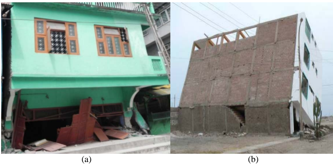
Fig. 1.4 (a) Failure of buildings due to irregular placement of infills during 2011 Sikkim earthquake; (b) ground story failure due to torsion effect during 2007 Peru earthquake (Johansson et al. 2007).
