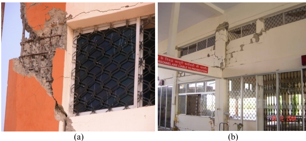
Fig. 3.3 Shear failure due to short column effect observed in Port-Blair, India, during 2004 Sumatra earthquake (Paul et al. 2004).
