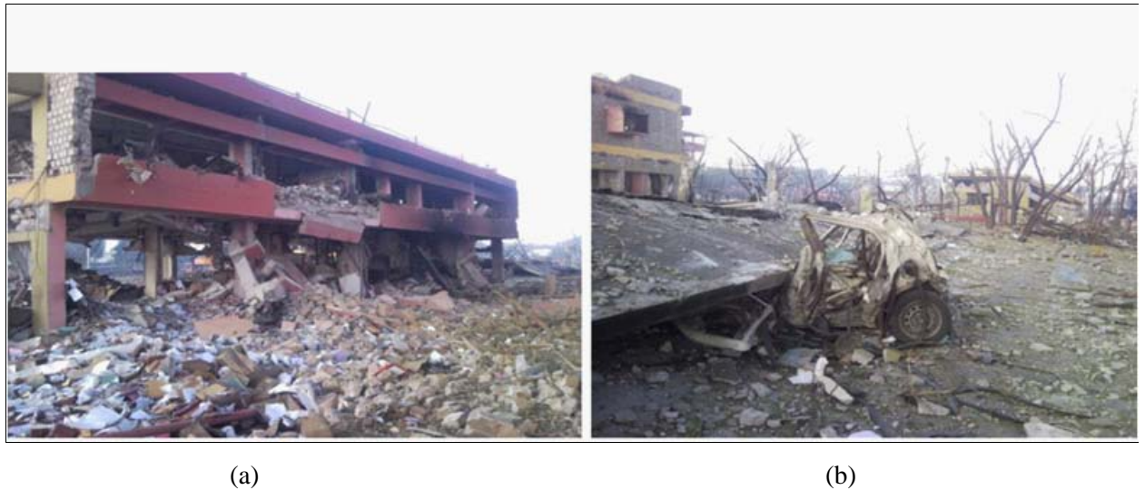
Fig. 4.6 (a) High level of over pressure damage at Terminal main building and (b) view of the damaged car parking
