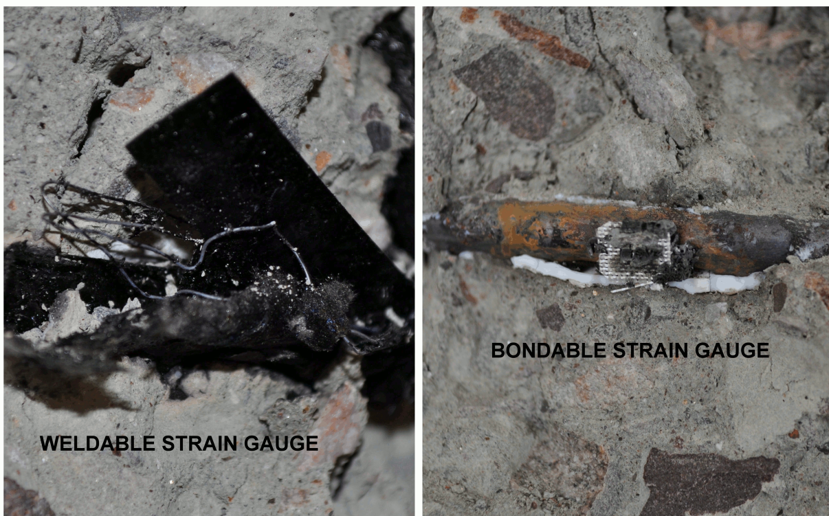
Fig. 3.18: Failure of Strain Gauges
