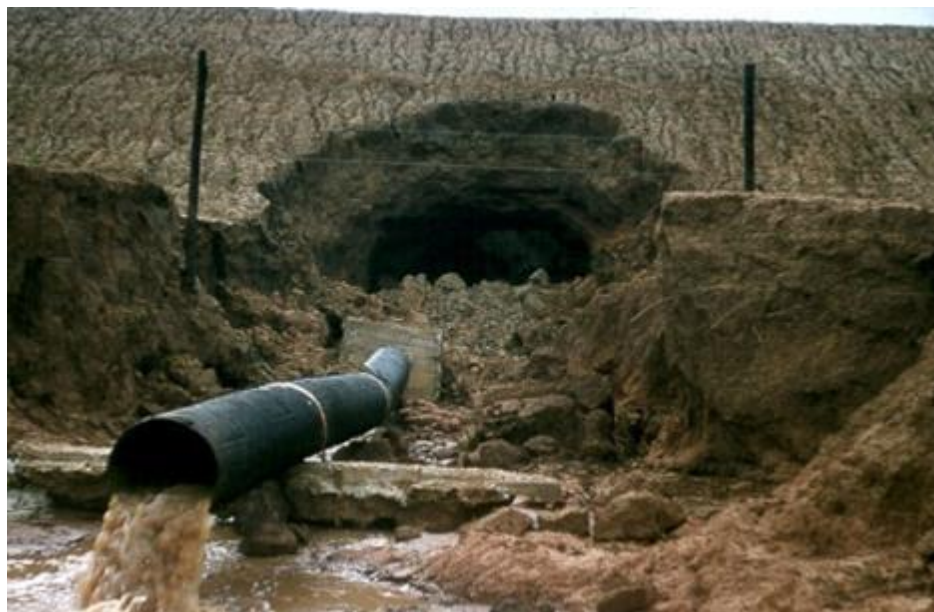
Fig.5 Embankment failure by piping along the outlet pipe (USDA, n.d.)
