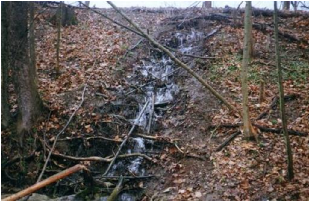
Fig.6 Example of seepage through an embankment (USDA, n.d.)
