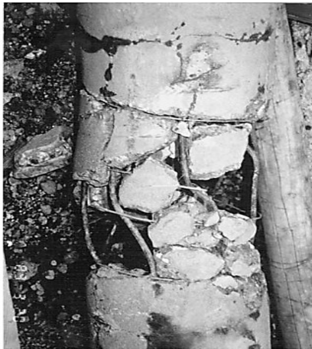
Fig.1.1 Damage of pile due to ground displacement Niigata 1964 [Finn and Fujita (2002)]
