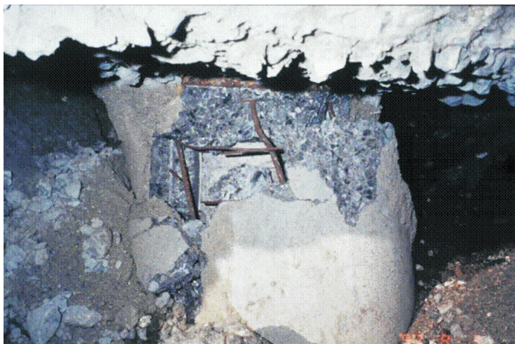
Figure 2.4: Damage at pile to pile cap connection due to strong earthquake, Teguh et al. (2006)
