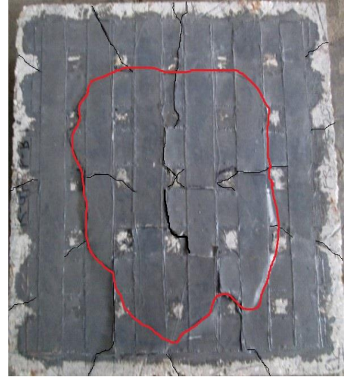
(b) Cracks on bottom face of RSG-70
