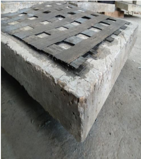
Figure 5.12 (a) Delamination of CFRP strips in RSC-70
