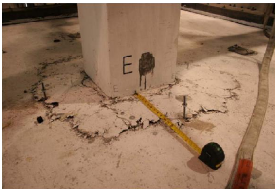
Figure 3.3 (a) Punching shear failure
