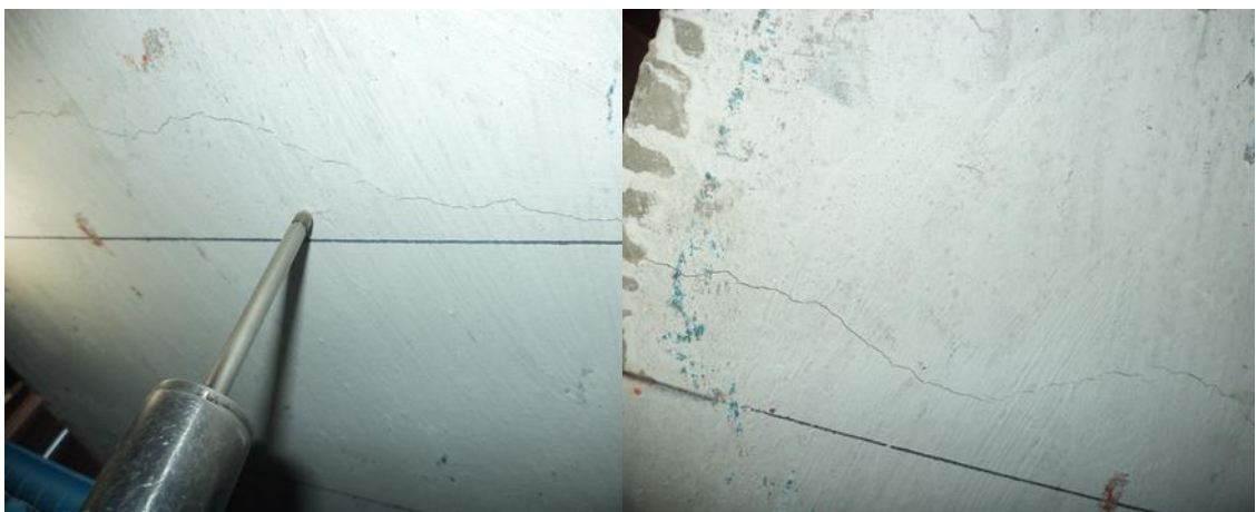
Figure 3.3: Cracks observed in flexural test at the mid-span and at the point of application of load
