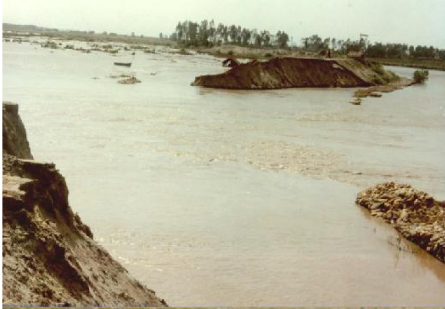
Figure 3.11 Embankment breach of railway track due to floods.
