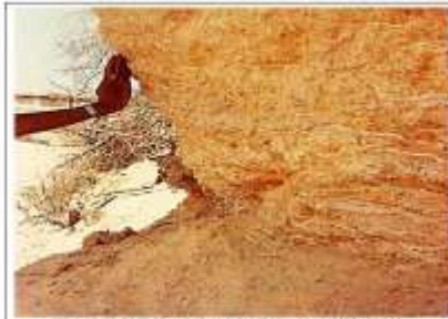
FIG. 1.28 CONTACT OF HARUDI SHALE WITH FULRA LIMESTONE NEAR VILLAGE HARUDI, IN BERWALI RIVER SECTION, SW-KACHOHH
