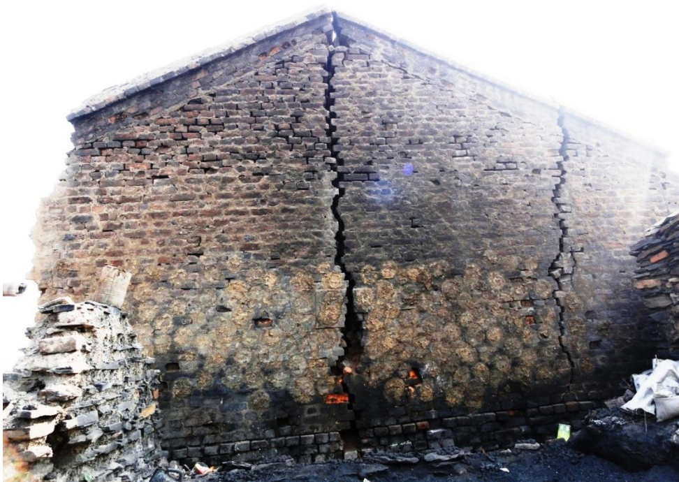
Figure 3.11 Shallow subsurface coal fires cause uncontrolled subsidence. The destabilization of land also causes damage to existing infrastructures. Here, massive cracks can be seen running through a main wall in the remains of a house. The longer crack is about 2.5 cm wide in most places (Prakash et al., 2013)
