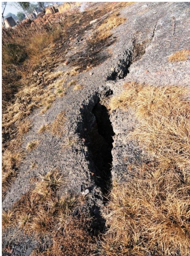
Figure 3.9 Development of broad linear crack of approximately 4 m in length and 5-15 cm in width. Degradation of vegetation is also visible. Such features are the surface manifestation of subsurface coal fire occurring underground (Bokapahari, JCF)
