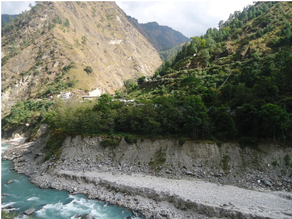
Fig. 8.27 Debris and RBM material present upstream of Urgam bridge on Left bank
