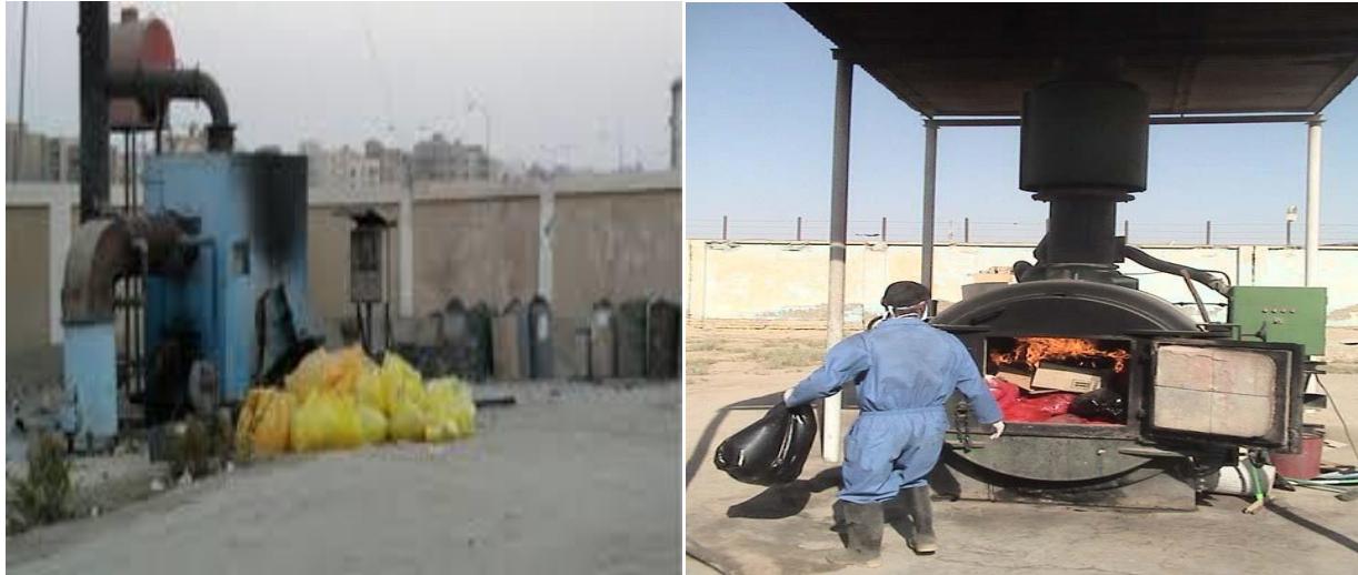
Fig 4.13: Incinerator Of Omdurman Hospitals
