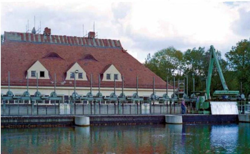
Fig 2.10:- Traversing Hydraulically Operated Trashrack Cleaner
