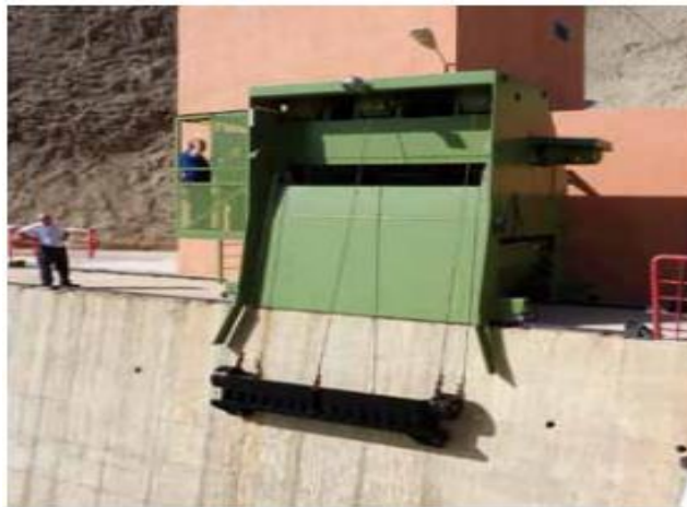
Fig 2.13:- Stationary And Traversing Cable Driven Trashrack Cleaner
