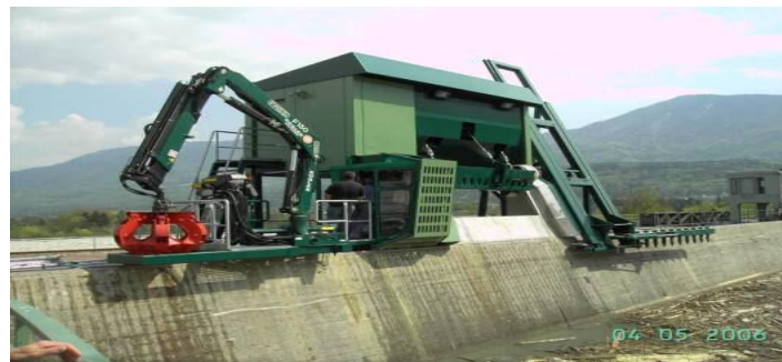
Fig 2.5:- Wire Rope Type Trash Rack Cleaning Machine (HPP Feistritz, Austria)
