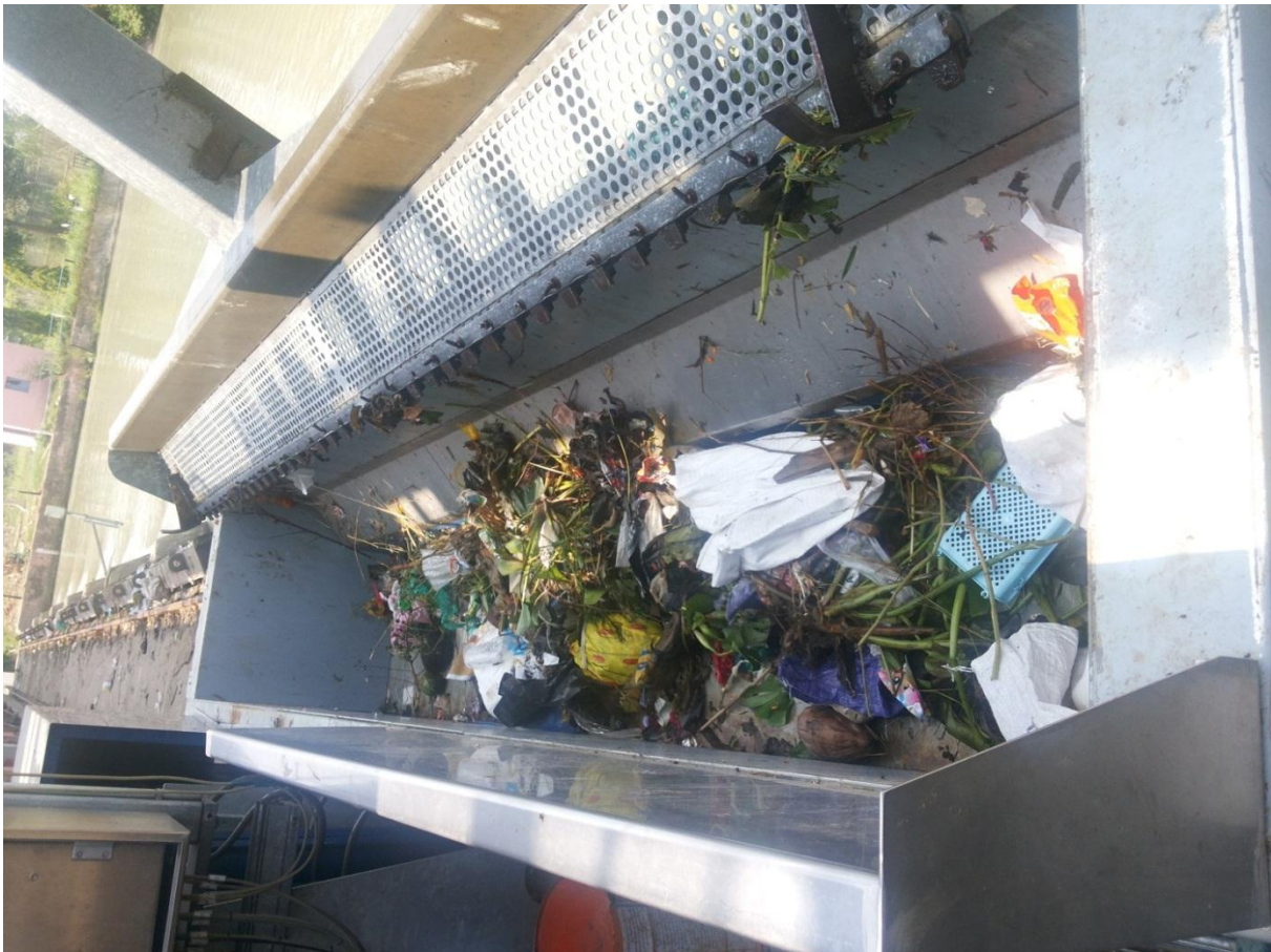
Fig 4.3-: Trashes Collecting Arrangement In Trash Rack Machine
