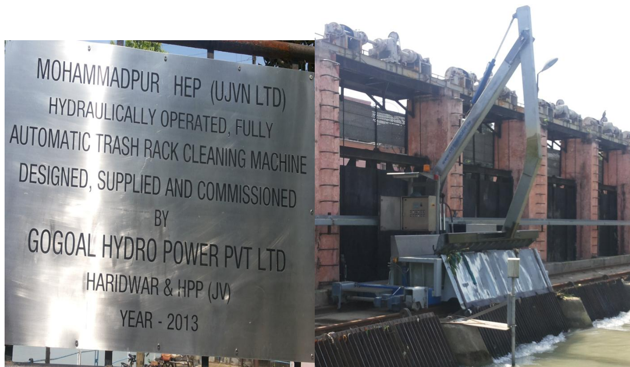
Fig 4.2:-Trashrack Machine At Mohammadpur Powerhouse
