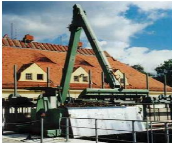
Fig 2.9:- Traversing Hydraulically Operated Trashrack Cleaners
