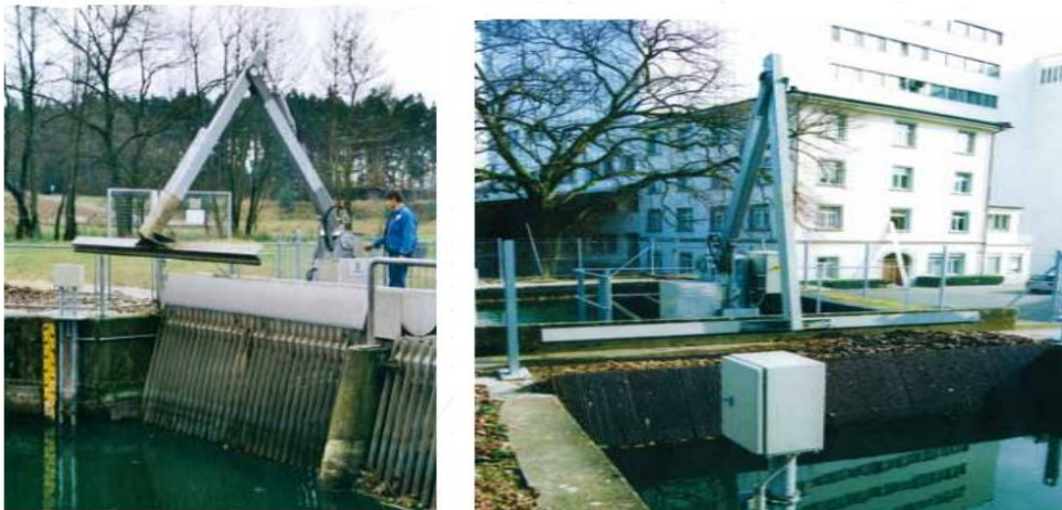
Fig 2.7-: Stationary Hydraulically Operated Trashrack Cleaners
