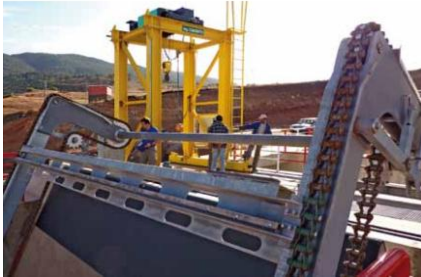
Fig 2.11-: Stationary Chain driven Trashrack Cleaners
