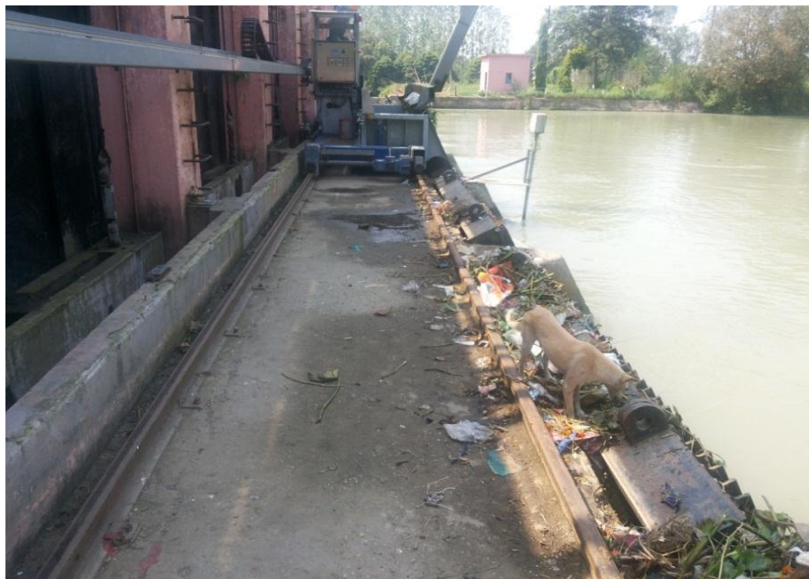
Fig 4.5-: Trashes Remain Above Trashrack after Cleaning
