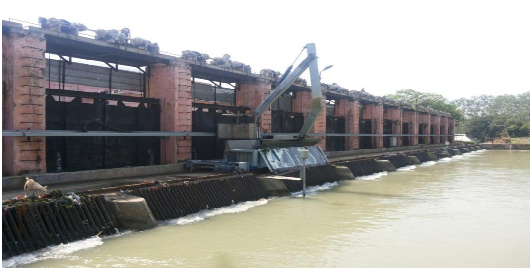
Fig 4.1:-Trashrack Machine in Operation at Mohammadpur Powerhouse
