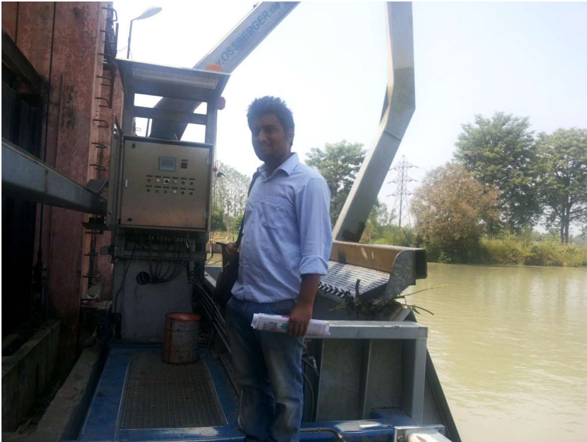
Fig 4.4-: Operation Panel of Trashrack machine
