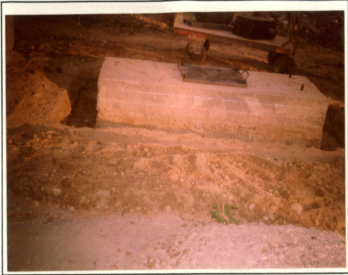
Fig. 15 A concrete block of dimension 2.25m x 0.75 m x 0.7m with base plate
