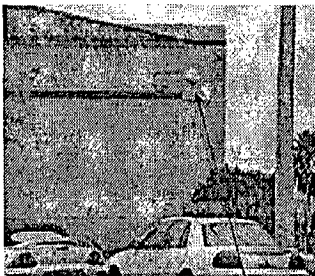
CCTV STRATEGICALLY POSITIONED TO MONITOR VISITOR PARKING AND BUILDING PERIMETER
