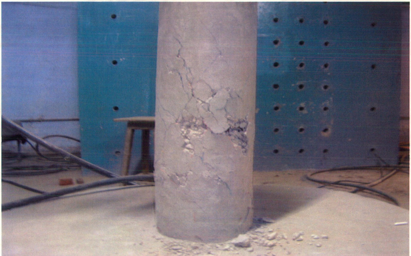
Plate 5.3 Spalling of Concrete in Model M1
