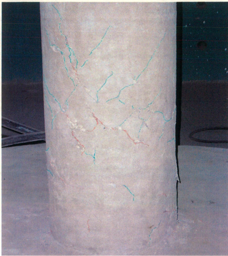
Plate 5.2 Cracks extended to mid height in Model M1
