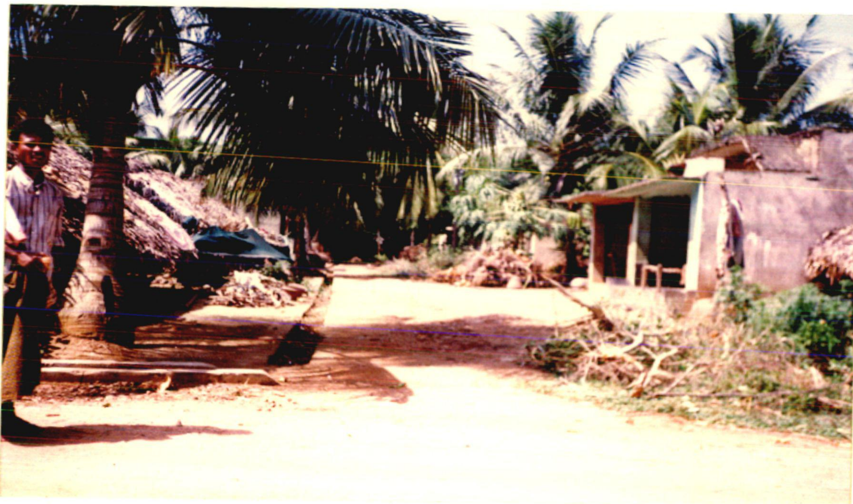
Fig 5.7: Non-functioning of the drainage system.
