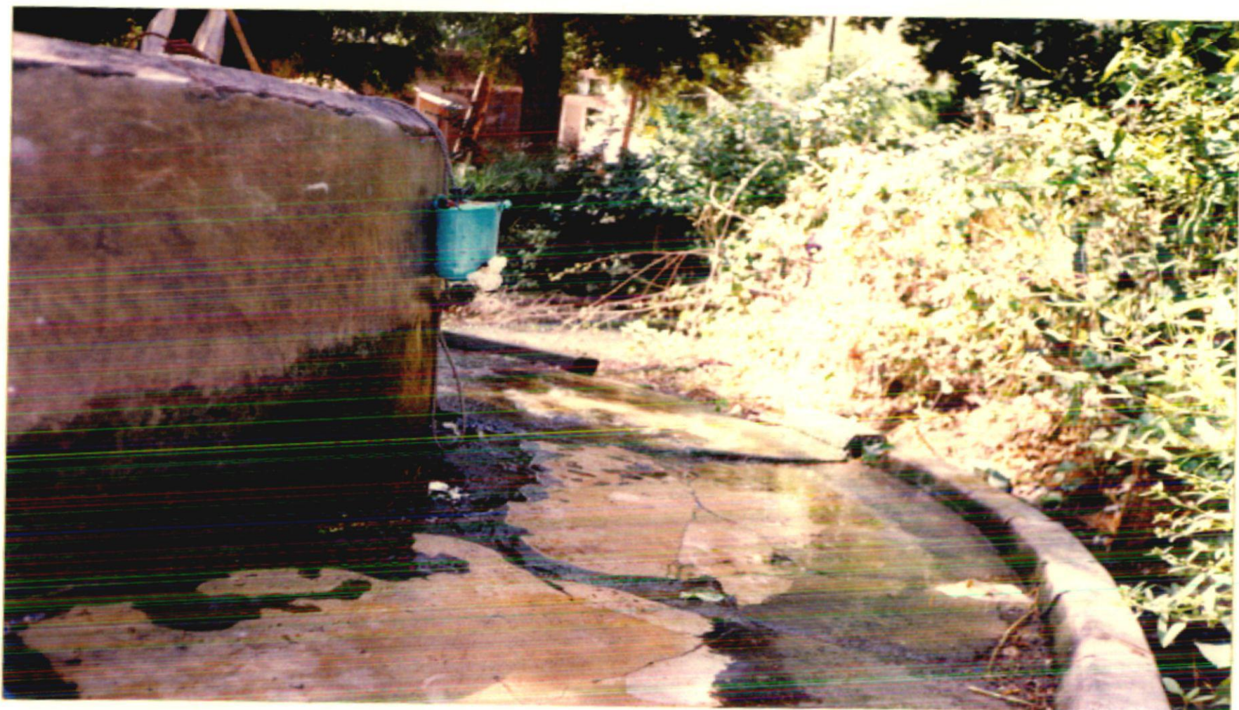
Fig 5.4: Unhygienic conditions prevailing at drinking water sources.
