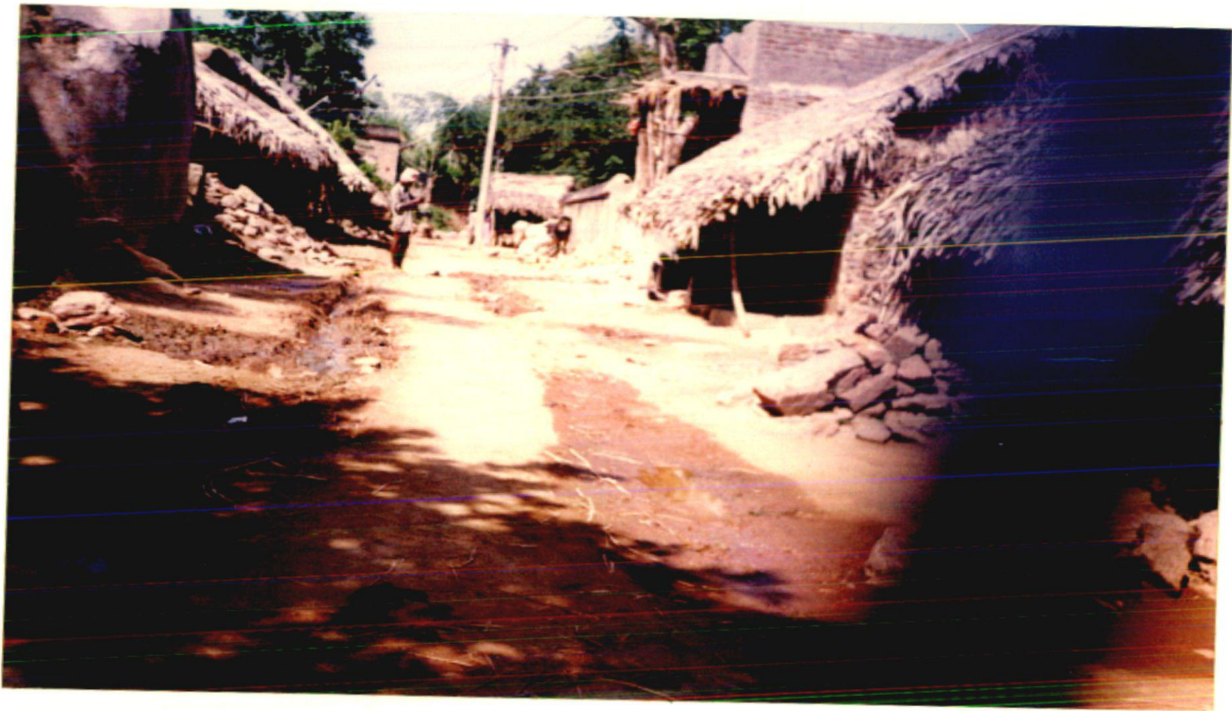
Fig 5.3: Poor condition of the only road in the village.
