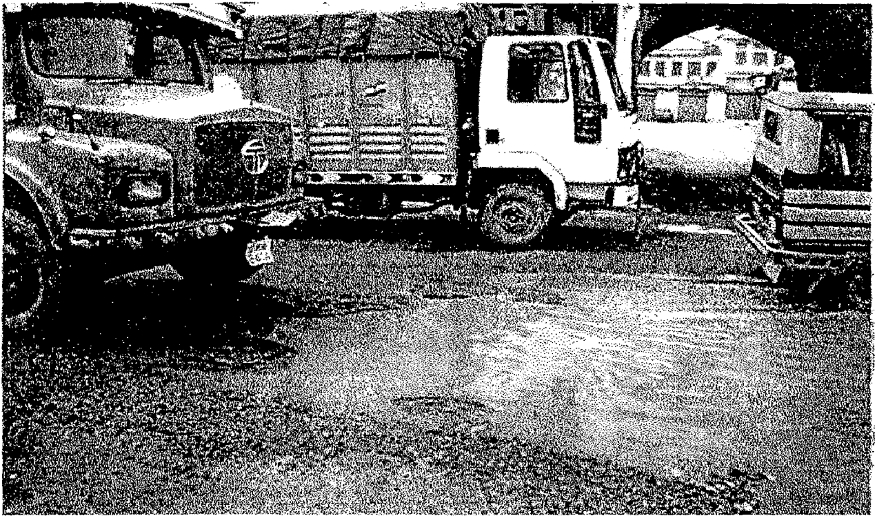
Poor Drainage Condition of the Main Road Reaching to main Tourist Centers
