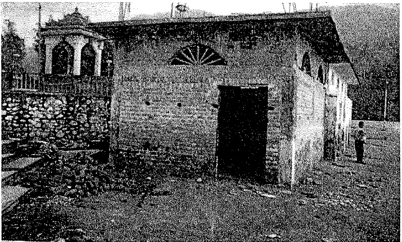
Poor Condition of Bathing Space at Treveni Ghat
