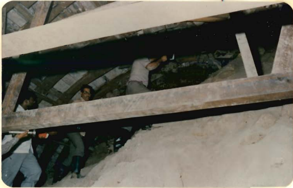
Fig.4.25 - A View of Collapsed Portion in Honnenahally Fault Zone (4th Collapse) of Bagur-Navile Tunnel
