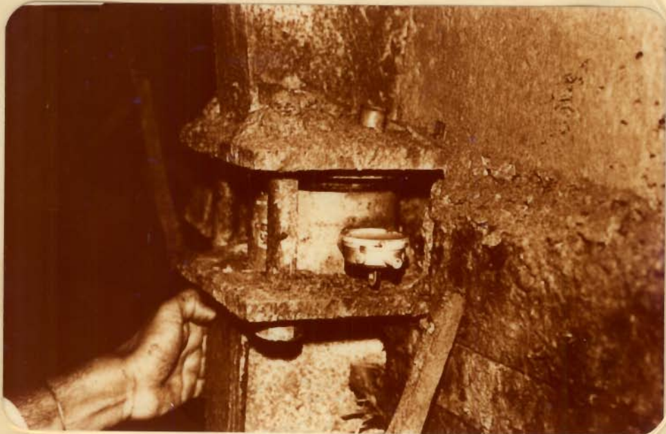
Fig.5.3(b) - A Mechanical Load Cell (with Dial Gauge) Installed within Steel Rib at Springing Level
