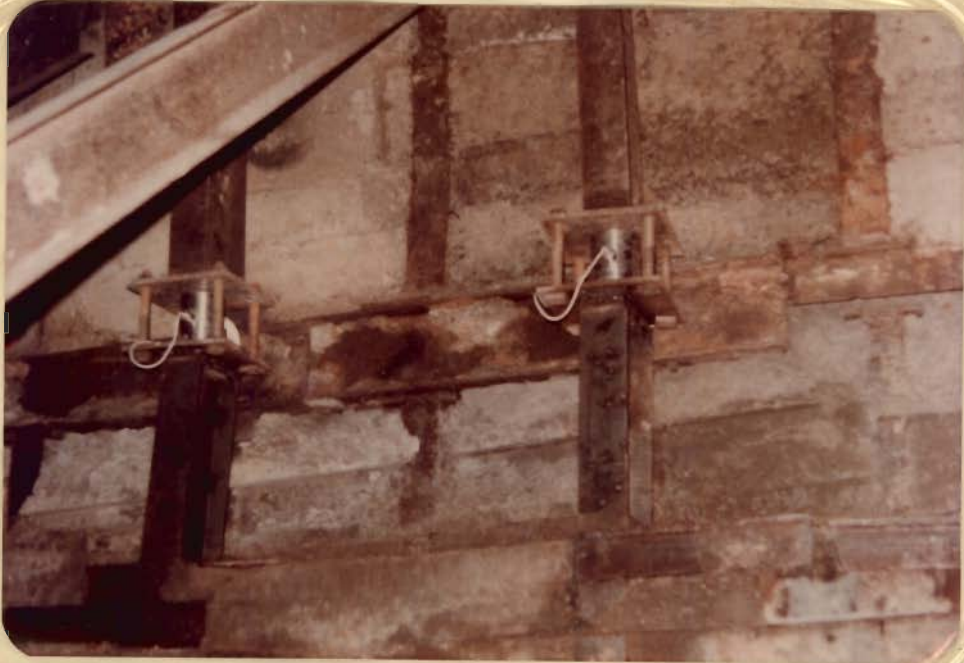
Fig.5.3(a) - Electrical Load Cells Installed within Steel Ribs at Springing Level
