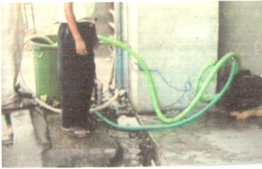
Fig. 5.66 direct pumping of Narmada Water
