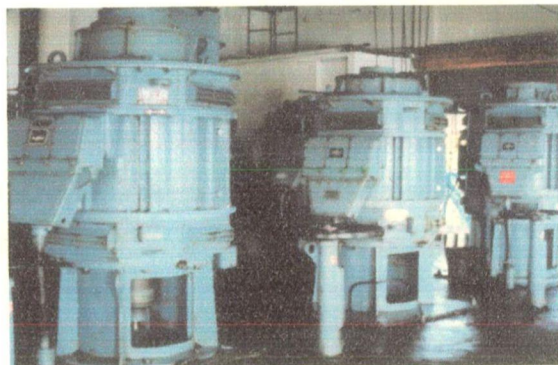
Fig. 5.58 Raw water pumps at Jalud
