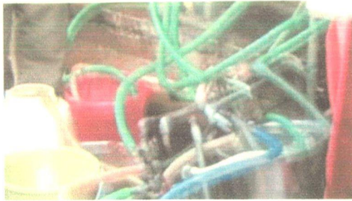
Fig. 5.67 A wrong manner of taking connection
