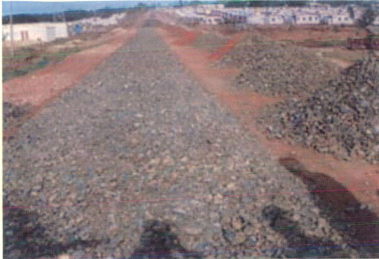
ILLUSTRATION 19: SNAP SHOWING ROAD CONSTRUCTION WORK IN PROGRESS AT MLTHAHALLI VILLAGE FROM STATE FUNDS
