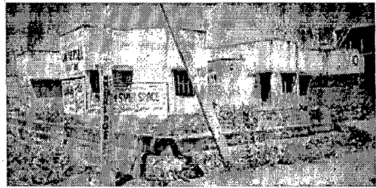
Fig 5.5g View shows the abandoned houses without compound wall causing intruders to enter.
