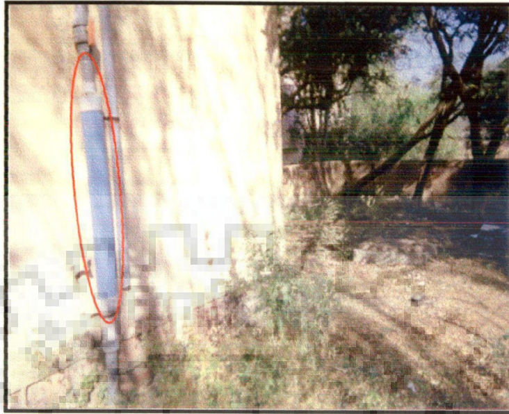
Plate 2.9: Vertically downward flow sand filter used for rooftop rainwater harvesting at Khandwa, India (Field visit)
