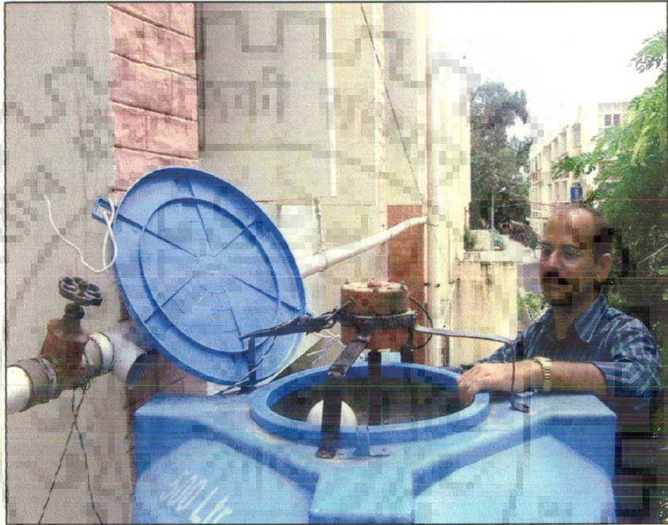
Plate 3.1: Overhead HDPE tank attached with stirring facility at I.I.T. Roorkee, Roorkee, India
