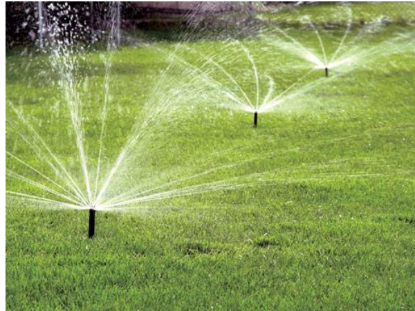
Fig. 5.2 Sprinkler System used in Lawns
