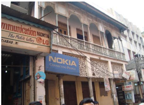
Figure 53 Left: Encroachments in Chopla area, Right: One of the narrow lanes, Source: Author
